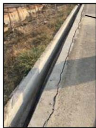
Longitudinal crack on landfill berm surface
