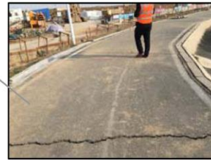
Transverse cracks on landfill berm surface at turning cover
