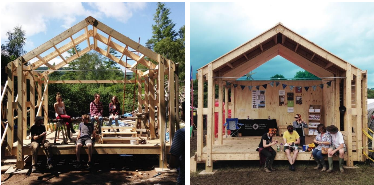
Figure 4.4: Prototype under construction at CAT and onsite in the Green Futures Field, Glastonbury
