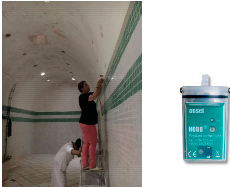
Figure 13. Installation of HOBO data loggers for measuring temperature and light: Temperature range: -20\text{ }^{\circ}\text{C} to 70\text{ }^{\circ}\text{C} , light measurement range: 0 to 320,000 lx (0 to 30,000 lumens/ft 2 ).
