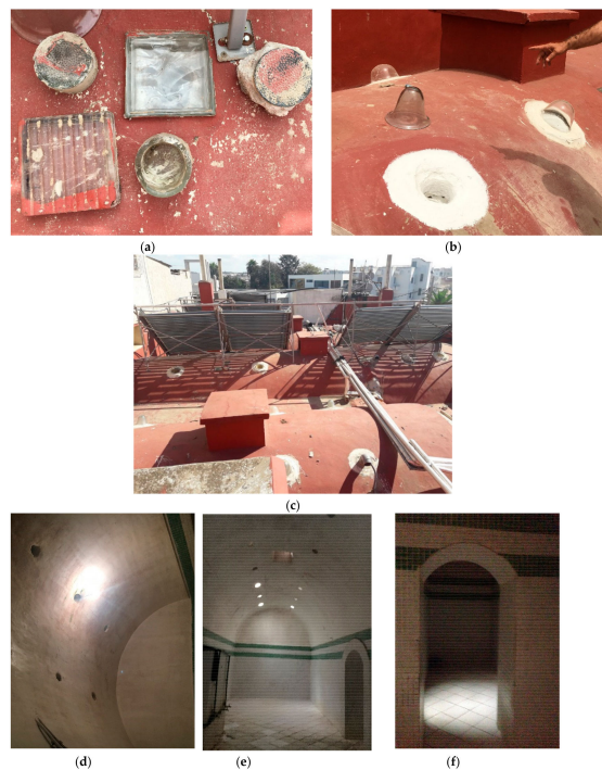
Figure 12. The roof of Hammam Rjafalla: (a) Removing poor alternatives of oculi covers; (b) re-opening the oculi and placing the blown recycled glass caps; (c) solar panels over the warm room affecting indoor daylight measurements; (d) blocked oculi in the hot room; (e) vernacular daylight restored; (f) oculi natural light effect.
