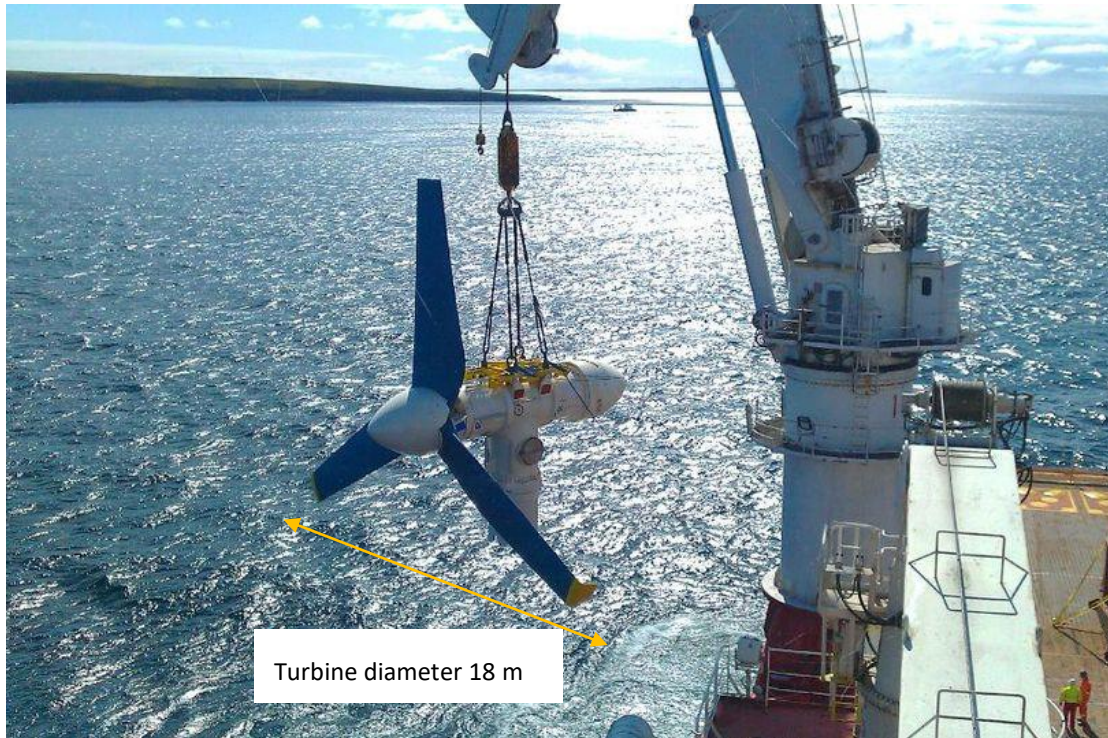
Figure 2-10 Atlantis AR1000 installation (Image Source: insider.co.uk)
