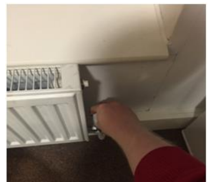
Figure 100. Using radiators in MH
