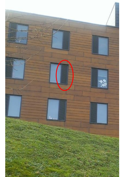
Figure 83. Louvers on MH room windows
