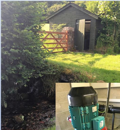
Images: Micro hydro 'house' and turbine
