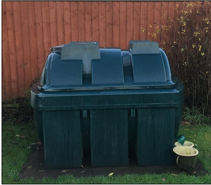
Figure 7.13. Outdoor tank used for oil storage Source: Author
