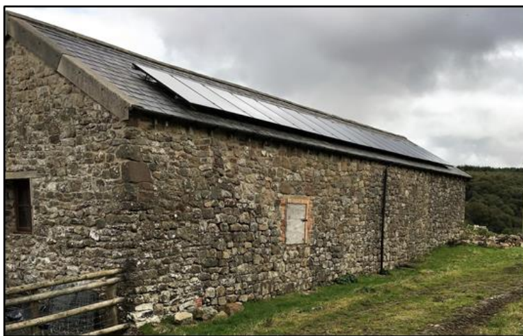
Figure 7.21. Roof-mounted solar-PV. Source: Author
