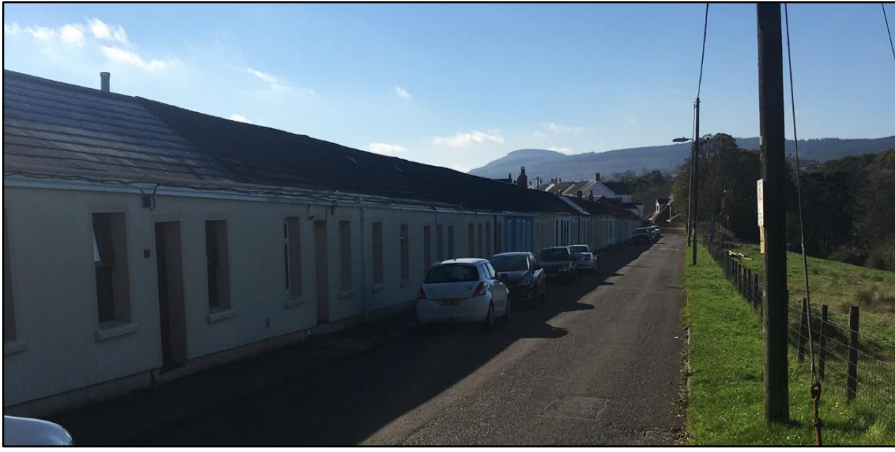
Figure 7.17. Row of stone-built terrace cottages (circa 1890s), most with external wall insulation cladding (mix of privately funded and Arbed). Source: Author
