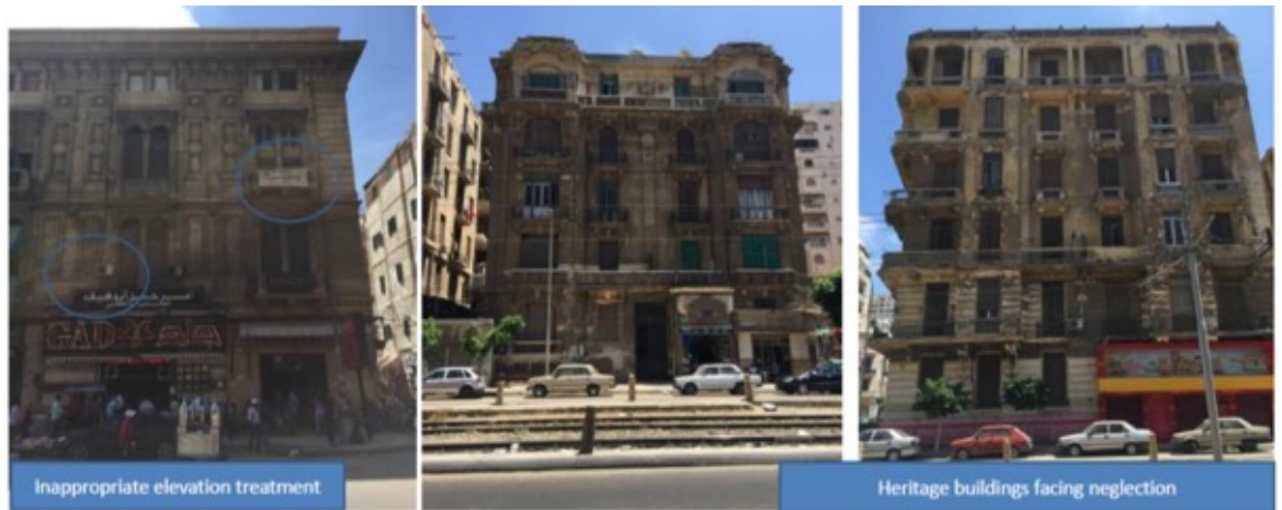
Figure 2-53 lack of maintenance and mal façade treatments
