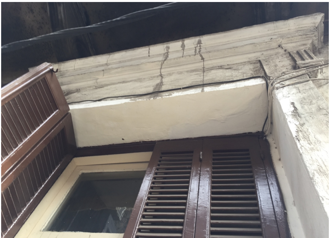
Figure 5-18 the openings lintels are supported by a concrete block hanged over the brick structure, source: the researcher
