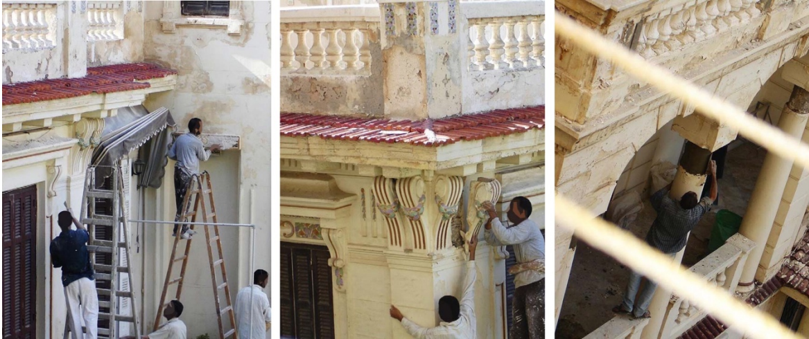
Figure 2-51 deforming the architectural character practices of listed buildings, from left removal or ornaments, removing moldings, and changing the column capital (Elsorady, 2011)
