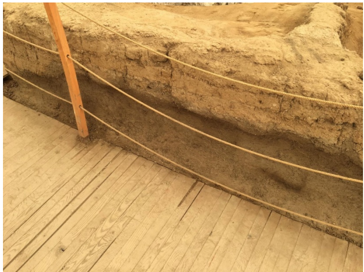
Figure 32: Wall repair on Building 64, undercutting support along the base of the wall. The area is first lined with geotextile, then layers of sieved earth mixed with perlite and chaff are applied to mitigate further erosion.
