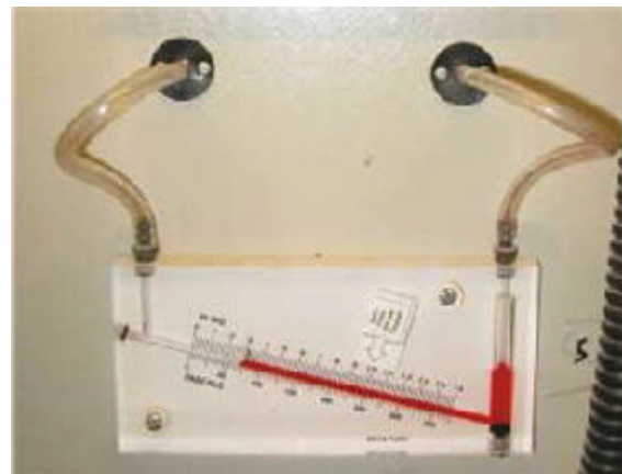
Figure 2. Label on manometer provides physical indicator of when to replace air filter due to increased pressured drop.
