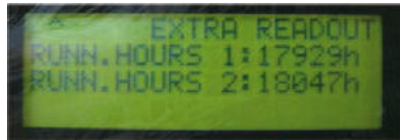
Figure 3. Compressors, Variable Speed Drives, etc. should have on-board diagnostics monitoring their running hours and other performance variables.
