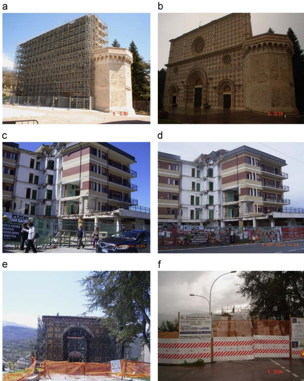
Fig. 5. Cases in the stages of the buildings. Progress in the reconstruction: (a) Santa Maria de Collemaggio (2010) and (b) Santa Maria de Collemaggio (2012) (inside is still propped). No changes between 2010 and 2012: (c) Student hostel (2010) and (d) Student hostel (2012). Buildings more deteriorated: (e) Porta Napoli (2010) and (f) Porta Napoli (2012). Photos by Diana M. Contreras M.
