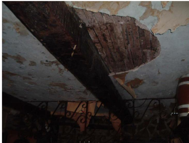
Photo 4. 8 Damaged pub ceiling
