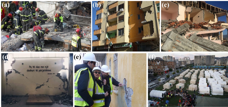
Fig. 2 Damages after the earthquakes in Albania on the 26th November 2019: a SAR operations after the earthquake; b Walls broken due to the earthquake; c Collapsed house. Source: Andonov et al. (2020a, b). d Broken wall due to the earthquake. Source: Watchman (2019) e The earthquake engineering field investigation team (EEFIT) checking structural damages during the earthquake reconnaissance mission. Source: EEFIT. f Distribution of humanitarian aid in a temporary shelter. Source: AITE-MIIE (2019)
