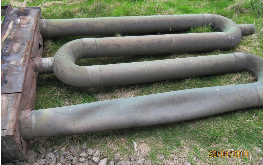
Figure 4-7 - A typical failure of Zodiac radiant tube. Deformation of firing leg, which in location, inside furnace, is the uppermost leg
