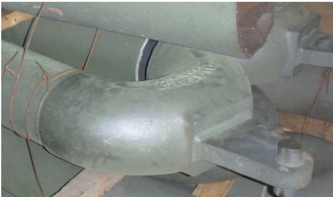
Figure 4-18 - Cracked radiant tube where weld are has failed
