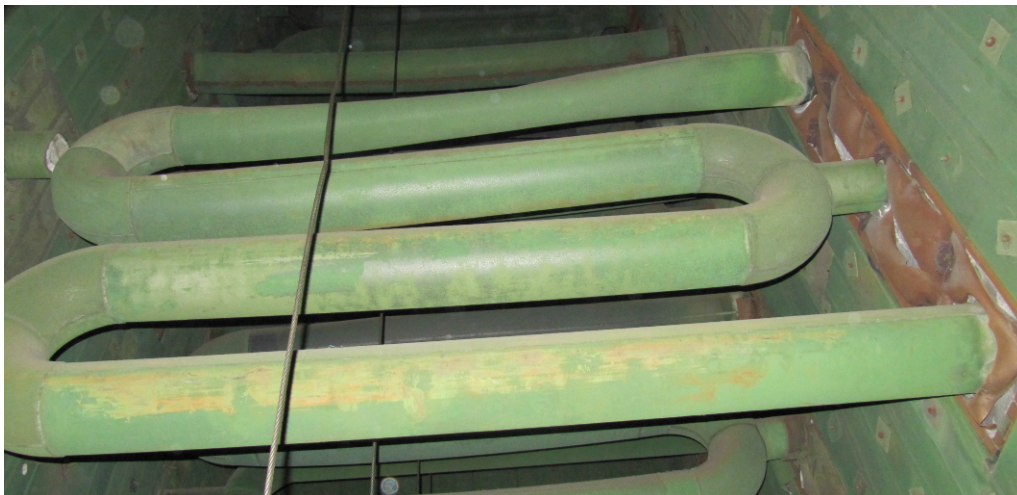
Figure 4-6 - A deformed firing leg in location inside furnace
