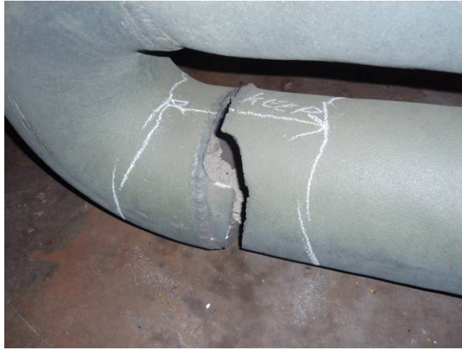
Figure 6-1 - Example of failure at weld region between firing leg and the first return bend
