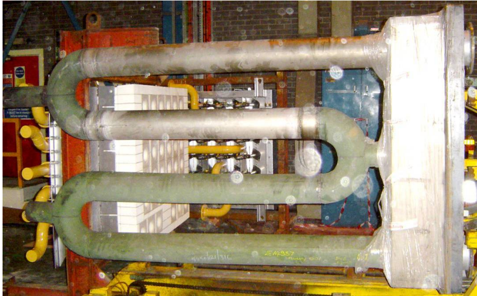
Figure 4-8 - A refurbished fabricated radiant tube used in the furnace of Zodiac, Llanwern.
