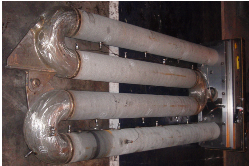
Figure 5-1 – Image displaying the radiant tube fitted with 20 thermocouples installed into zone 7 of the furnace for data acquisition
