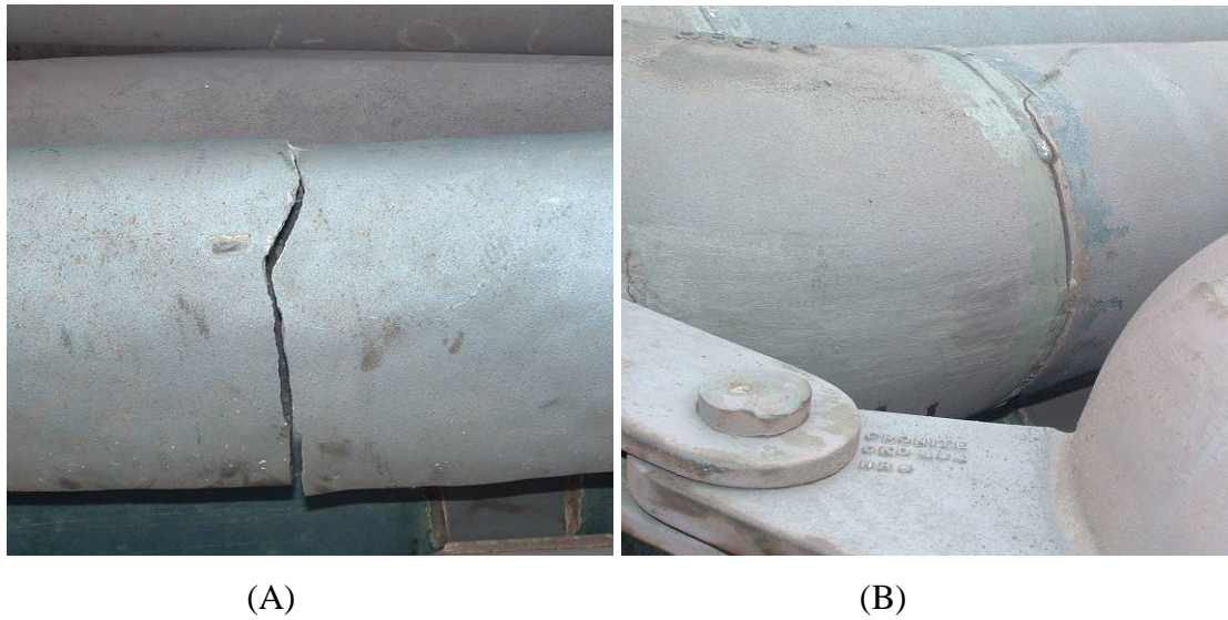
Figure 4-2 - Pictures indicating the common failures of tubes at Trostre; (A) cracking of the firing leg and (B) of the weld region of the 1st return bend
