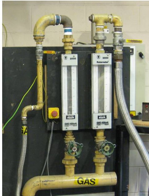
Figure 8-4 - Natural gas rotameters to indicate pilot gas and main burner gas flows (L/min)
