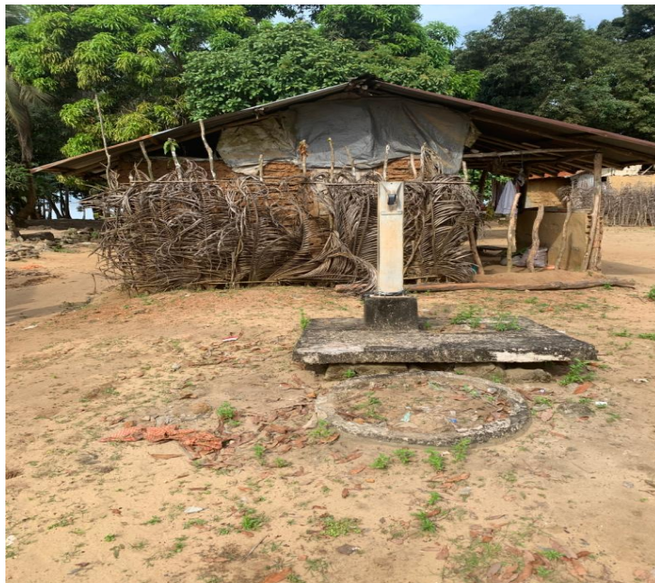
Picture 3: Damaged Hand Pump in Latia Town, Lake Piso Multipurpose Use Reserve Protected Area, Grand Cape Mount County
