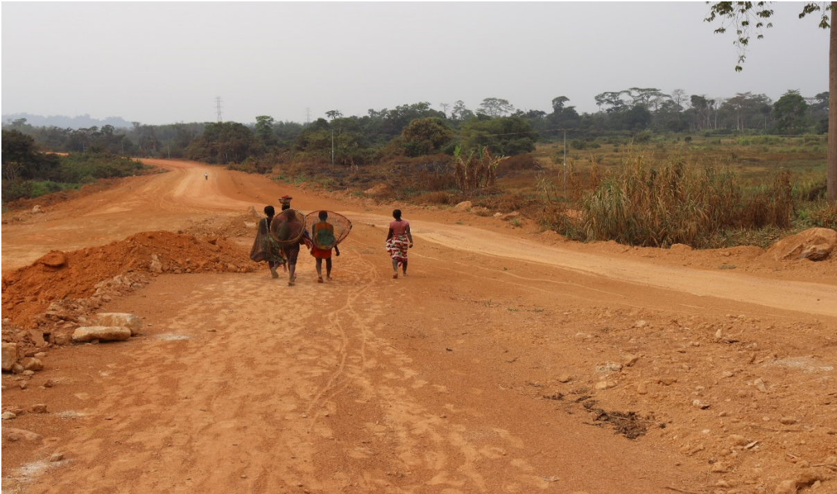
Picture 18: Road grading work on section of the Ganta-Sanniquellie - Yekepa Road in February 2020
