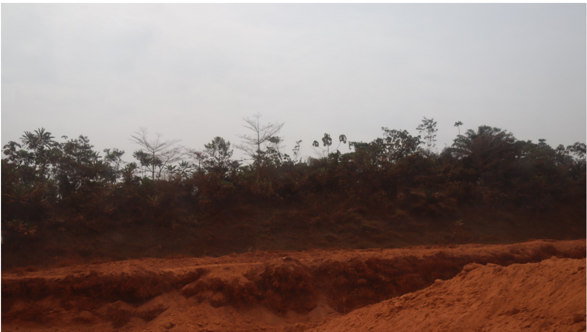
Picture 17: Collapsed Section of the Ganta -Sanniquellie-Yekepa Road (little dry in February 2020)
