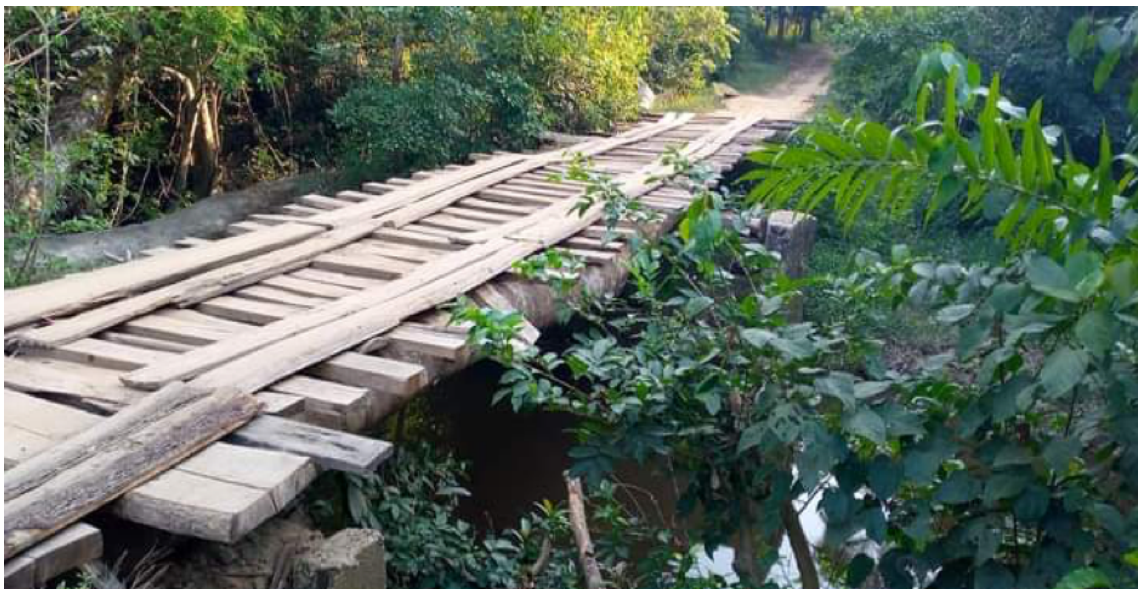
Picture 15: Abandoned SDF project, Baryata Bridge Project, Gbarlorkpala, Kokoyah District, Bong County, Liberia
