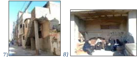
Figure 14: Violations on residential streets in the Baqaa camp. source author.
