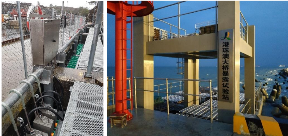
Figure 1: Austefjord field station supported by an existing quay, Norway (left) and HongKong-Zhuhai-Macau Bridge exposure site built into the project, China (right). The exposure sites may be built on some existing structures, such as wharves in service, or designed and built as new structure. In either case, the service life of the structures should cover the expected operation duration of the exposure site. Courtesy of Dr. Karla Hornbostel (Norwegian public roads administration) and Mr. Yan Yu (HZMBA).
