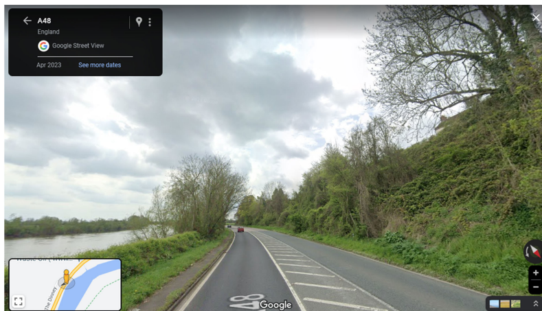
FIGURE 12. The embankment corrected by the Bayesian model in the flat region (© Google, 2023).
