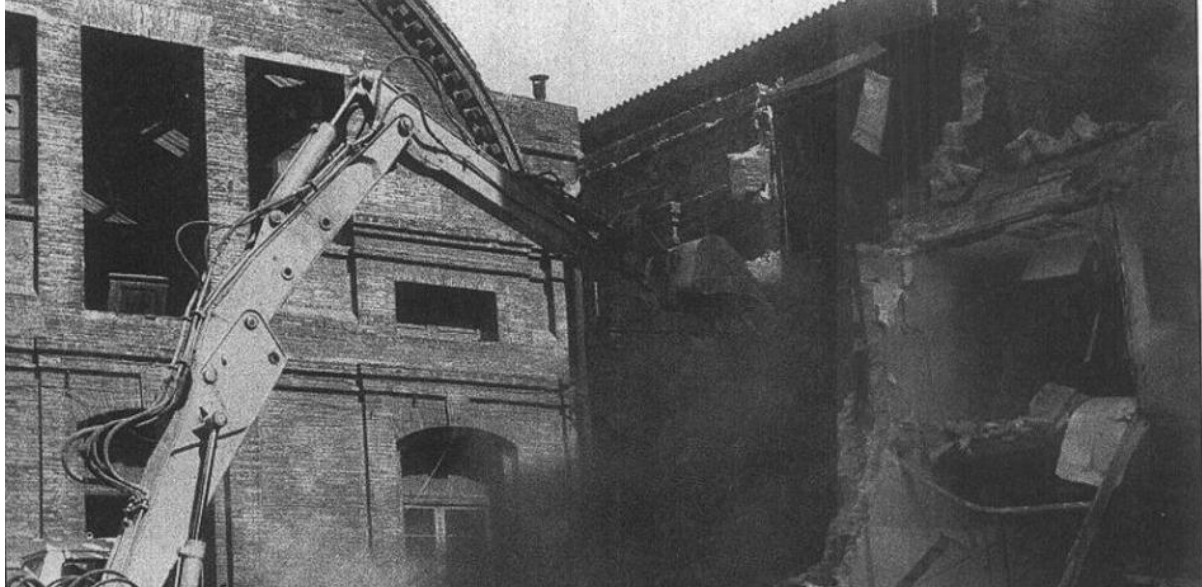
Figure 5.5: Manresa, K. (1987) Beginning of the demolition works in Icaria on the 3rd August 1987. The photograph taken in 1987 clearly indicates that some demolitions in the area had commenced prior to the commission in 1988 of the report of buildings slated for destruction by the Archaeological Department of the Museum of History of Barcelona-MUHBA (Source: La Vanguardia Newspaper Digital Archive). Available at 30 años de la destrucción del barrio de Icaria, la actual Vila Olímpica (lavanguardia.com) . (Accessed: 21 July 2020)
