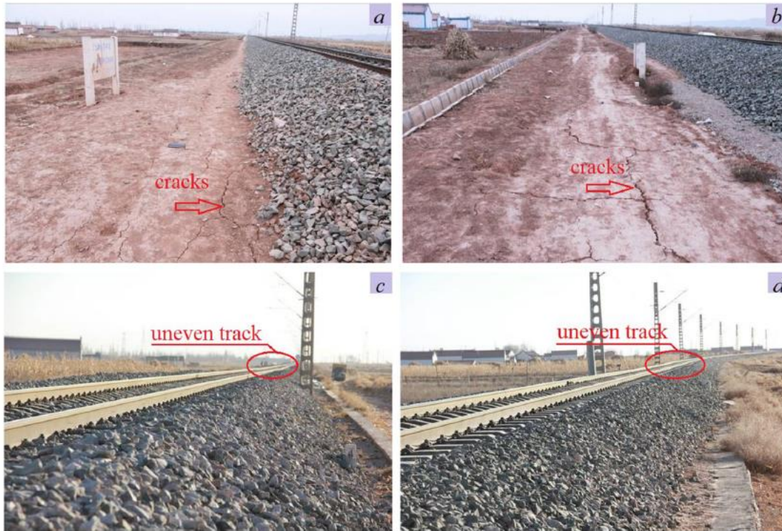
Fig. 3 Subgrade disease of Baozhong railway. a Cracks at K330+000 section; b Cracks at K330+200 section; c Uneven track at K330+200 section; d Uneven track at K331+250 section.
