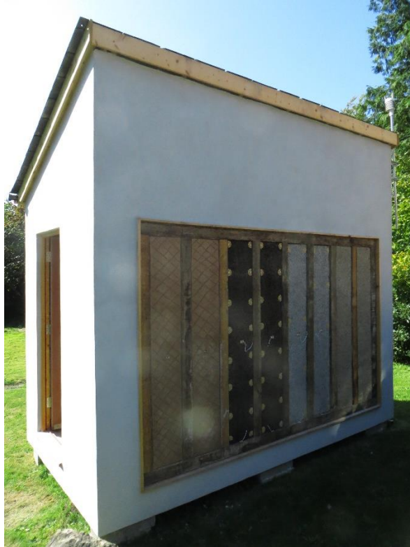
Figure 2. Test cell showing north façade prior to application of external render. Panels left to right, wattle-and-daub, expanded cork board, wood fibre/wood wool composite and hempcrete. Source: (Author's own, 2019)
