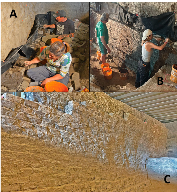
Figure 9. The mudbrick retaining wall and sacrificial facade in Section I, showing A) the authors laying down the first course, B) the wall nearing completion, and C) the completed facade after drying.
