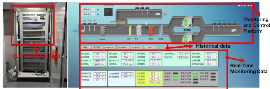
Fig 2. System control cabinet (left) and monitoring (right)
