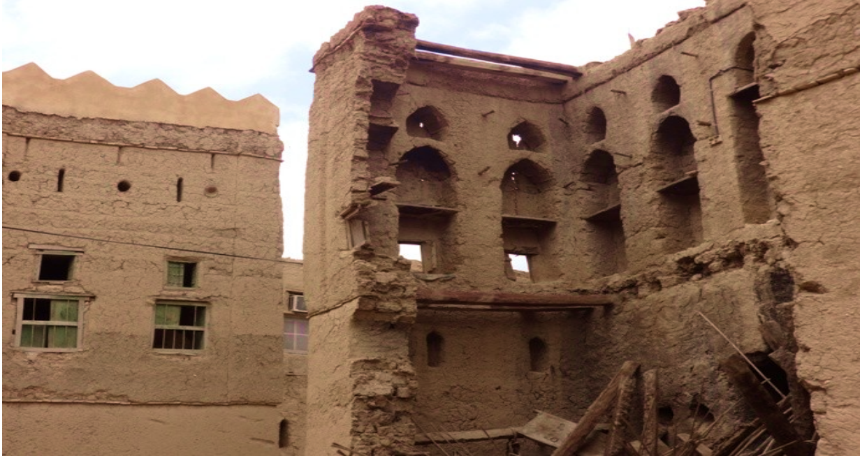
Picture 3.1. Omani heritage house built with Sarooj, wadi stones, and date palm trunks. Picture attribute Bait Al Safah Museum.
