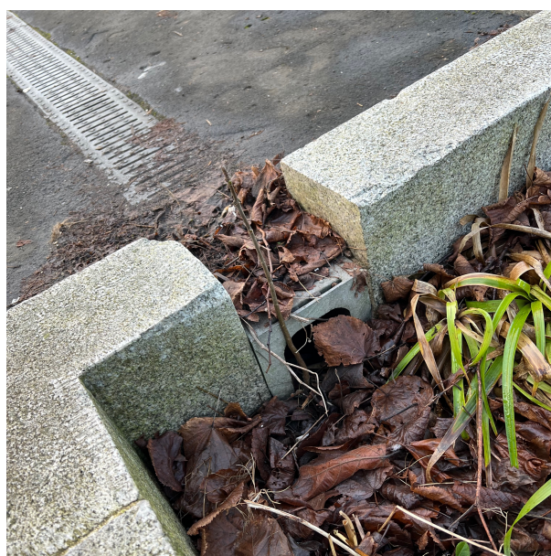
Figure 6.8 Channel inlet configuration of the biofilter located at the junction of Clydach St., Grangetown.
