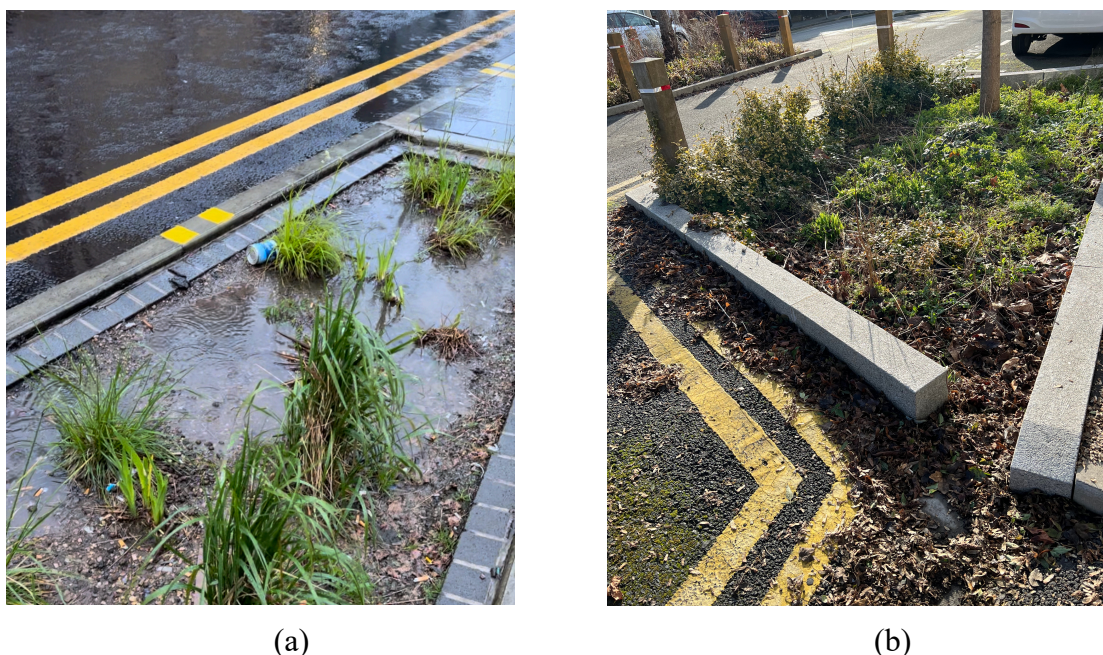
Figure 6.3 biofilter inlet design, (a) diffused inlet in Station Terrace biofilters, (b) centralised inlet in Greener Grangetown biofilters.
