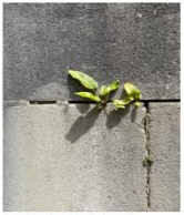
21. Vegetation growth through mortar joints
