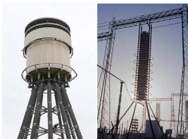
Fig. 2.15 HVDC Smoothing Reactor and DC-filter with capacitor [42].
