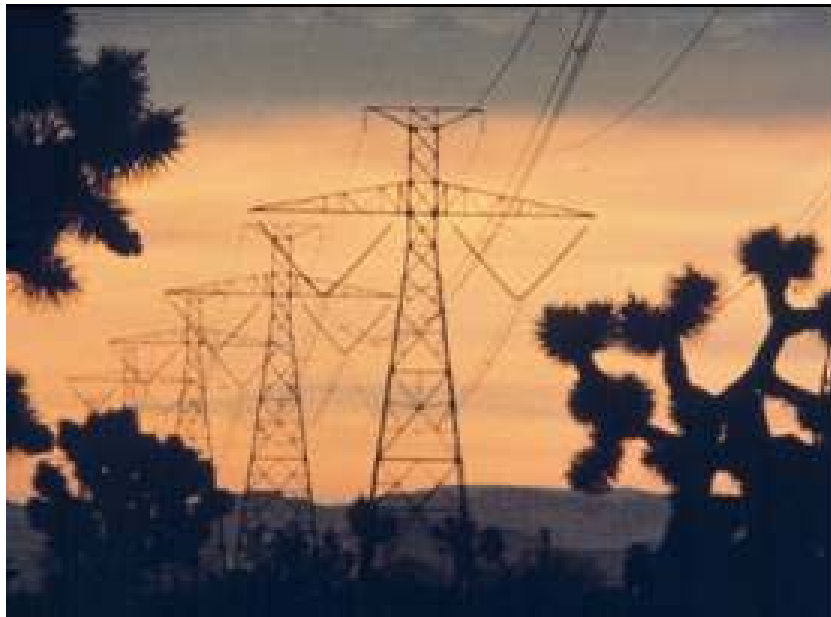
Fig. 2.1 \pm 500 kV HVDC transmission line [36].
