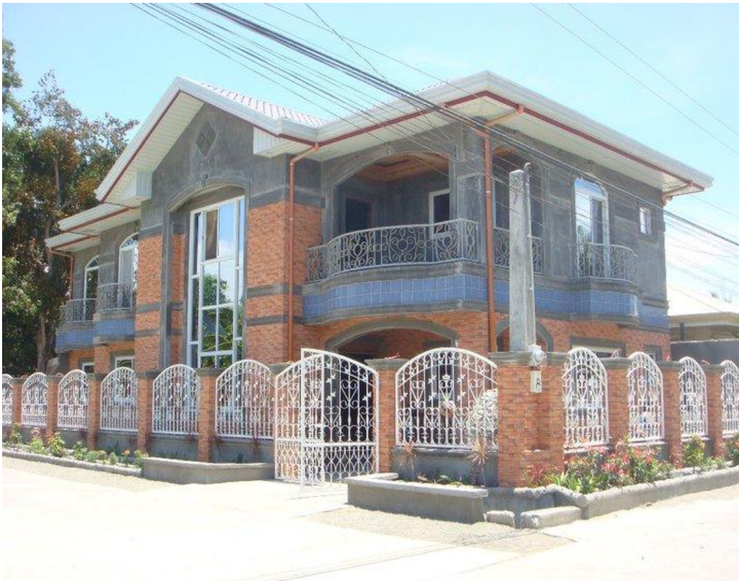
Figure 4.6 House of an overseas contract worker, San Gabriel. Work on-going. Photo used with permission of owner.
