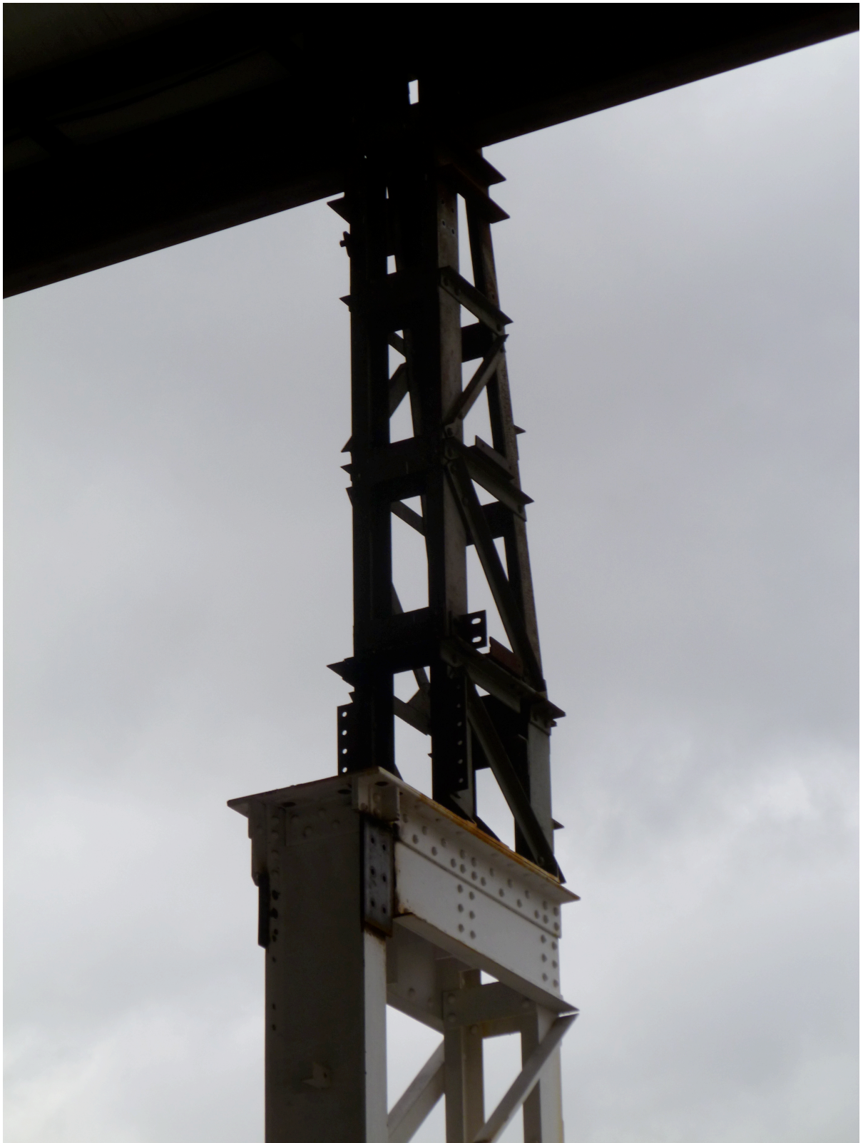
Existing composite columns and steelwork was preserved and used to carry the new energy producing envelope
