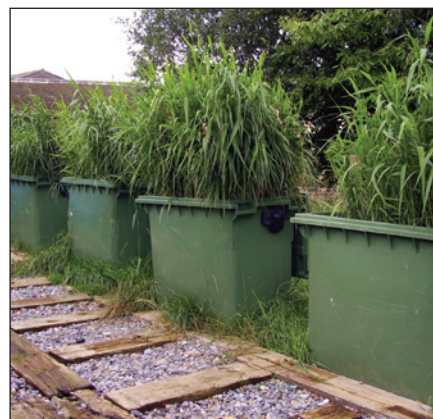
The pilot-scale alum-sludge-based engineered wetland wastewater treatment system at an animal farm in Ireland has cut soluble reactive phosphorus by up to 99.8% and BOD 5 by up to 90%
