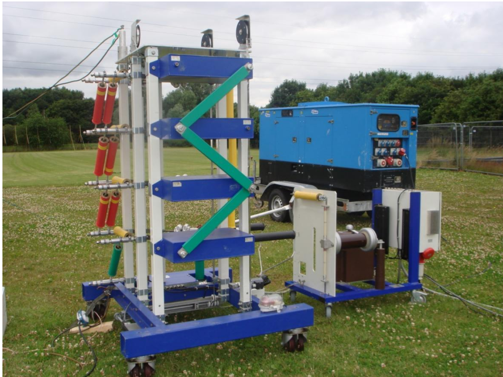
Figure 5.2: High voltage current generator at the field site
