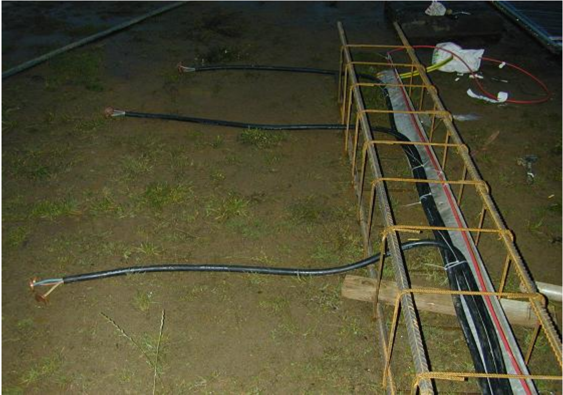
Figure 3.20: Preparation of probes in soil at different depths and 1m distance from footing No. 2 for measurement of potential (pre-installation)
