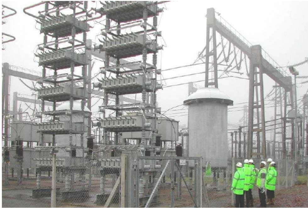
Figure 2.15: MSCDN installation at 400 kV operational substation in the UK [2.25]
