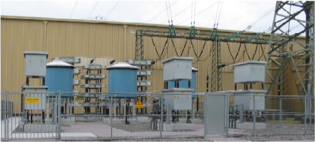
Figure 2.19: C-type filter installation rated 150 MVar at 220 kV [2.32]
