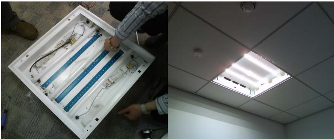
Figure 7.1 Combined fluorescent and LED luminaire. The LEDs are placed on three blue coloured modules (left image). LED lighting turned on and in use (right image). (Note: for demonstration purposes the light diffusing panel in front of the luminaire was removed)
