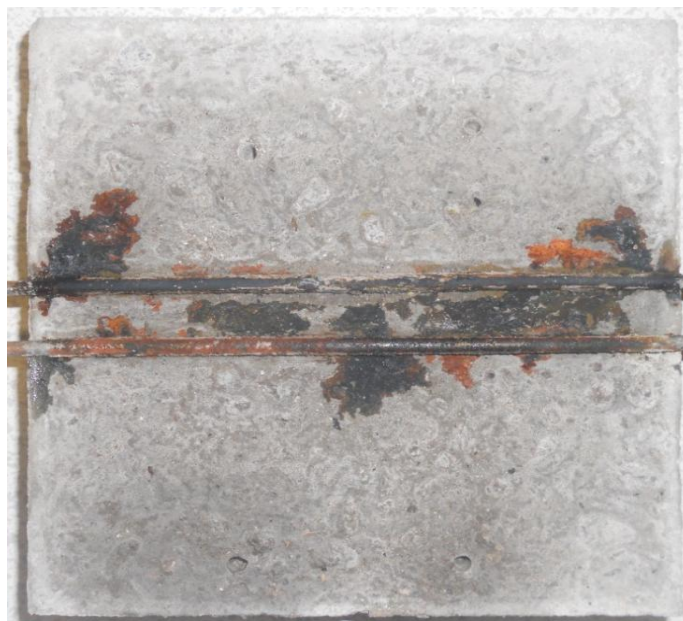
Figure 4. 41 Photograph of upper concrete surface and wires
