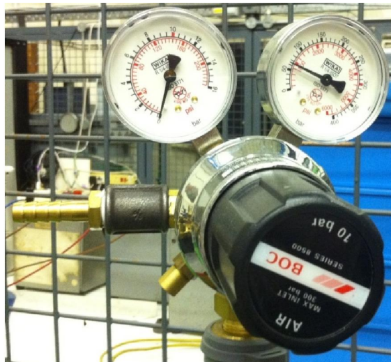
Figure 3.14: Compressed air pressure regulator
