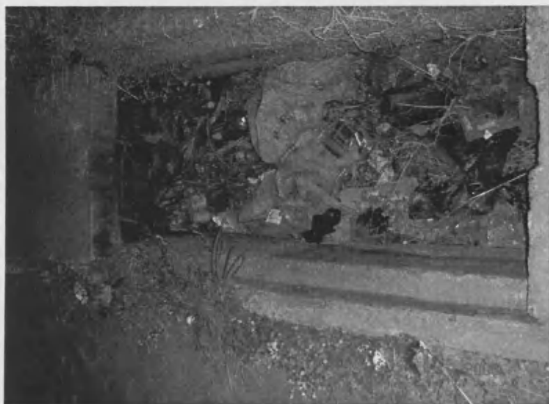
Picture 9.3: A water drain filled with waste
