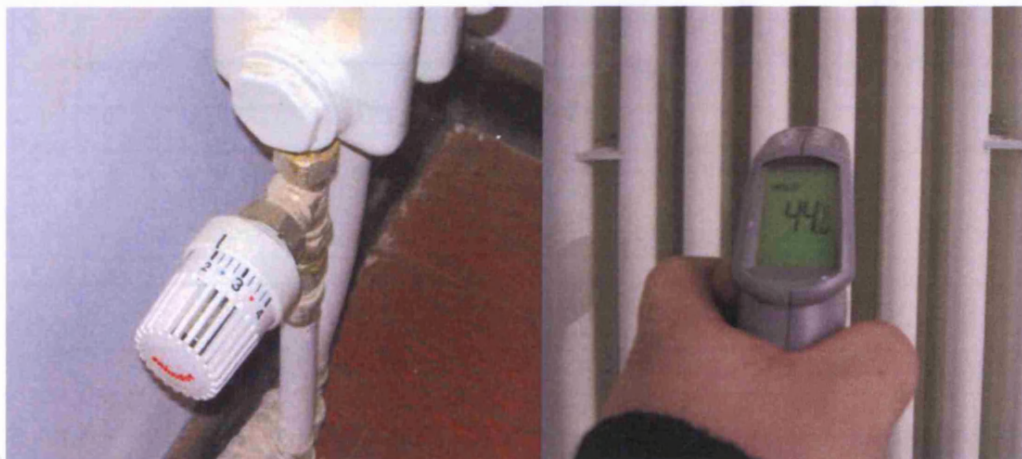
Figure 5. 31: Central Heating System was in Operation and Switched to Same Level
