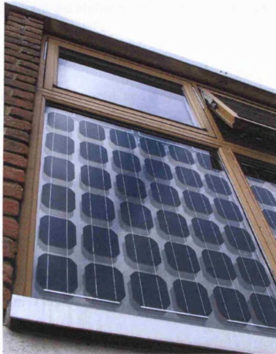
Figure 7.23: PV Cells on the Window, the BedZed project. Source: Author
