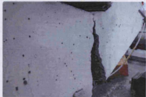
Figures 5a and b above: Beam failed in shear mode and flexural mode.
