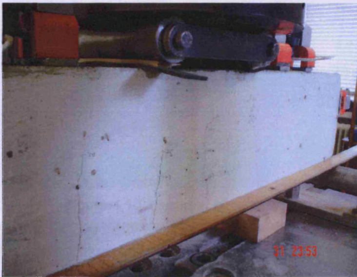
Figure 4.8: Distributed flexural cracks.
