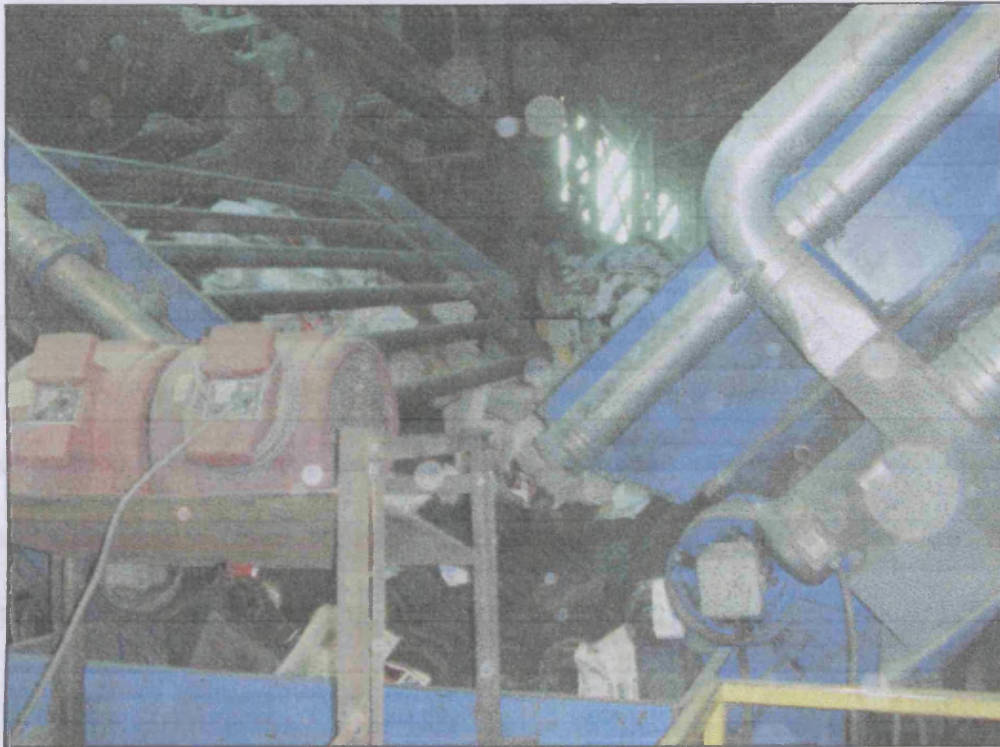
Figure 4.7: V-Screen at Blue Mountain Recycling MRF
