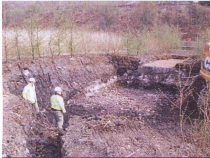
Figure 4-11: Looking east across the finished excavation ready for delivery of Type 1 sub-base.
