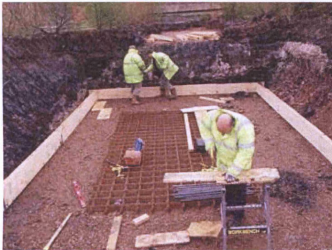
Figure 4-12: View facing east of the assembly of the ply-wood shuttering, ready for layering of the reinforced mesh and concrete pour.
