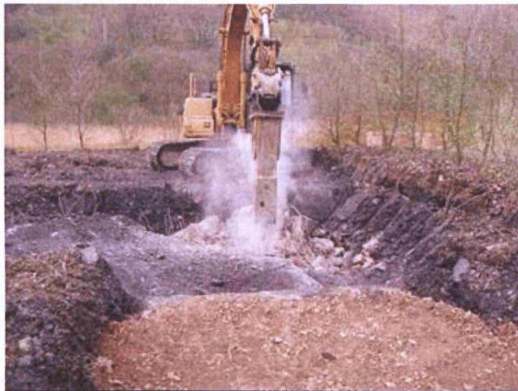
Figure 4-10: View looking west across the excavation showing the use of the pneumatic hammer to break the reinforced concrete slab.
