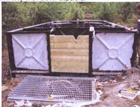
Figure 4-22: View looking east of the finished discharge chamber showing the galvanised steel grating.
