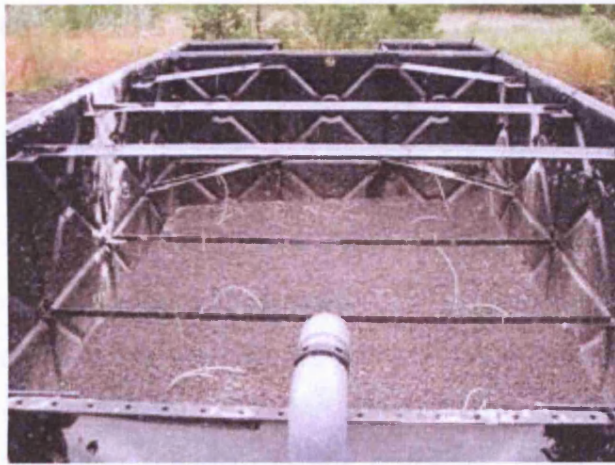
Figure 4-18: View facing west of the finished plenum floor with the 100 mm thick bed of 20 mm sandstone gravel.
