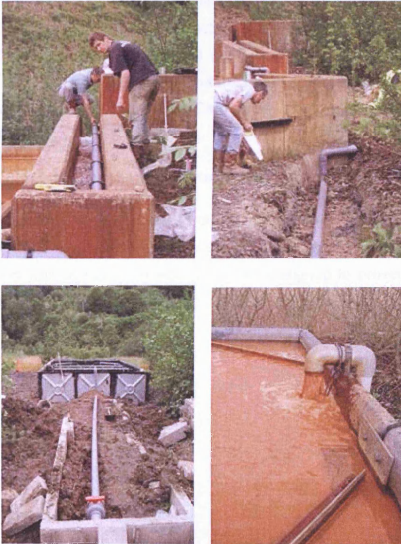
Figure 4-24: Sequence of photographs showing the feed pipe from the distribution weir to the VFR inlet
