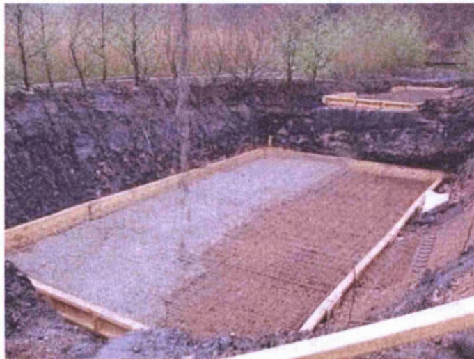
Figure 4-13: View facing east during the first pour of concrete onto the sub-base, shuttering-mesh assembly.
