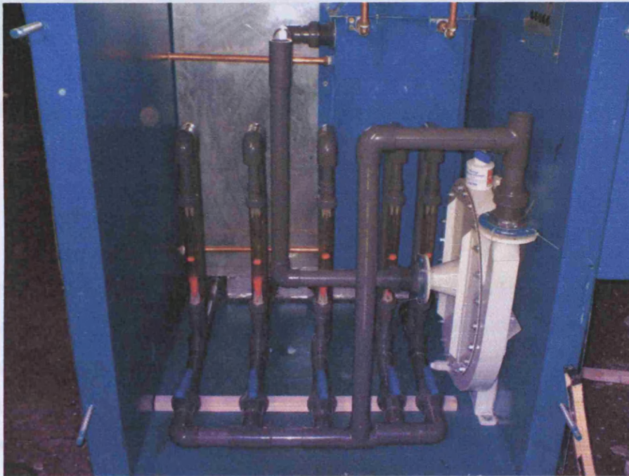
Figure 5.3 The recirculation pipe work and fan mounted in one half of the insulated vessel ( the fan is on the right, manual valves controlling flow into each part of the plenum floor are in the fore ground and rota-meters measuring flow into each part of the plenum floor are mounted vertically in the centre).
