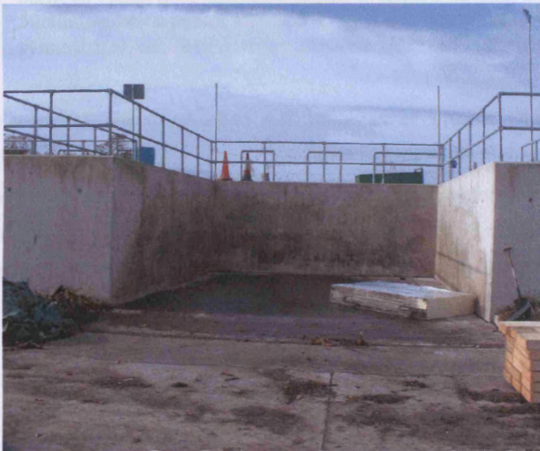
Figure 4.1. Concrete constructed bay in which the composting trials were conducted, 6 meters wide, 7 meters long and 2.2 meters high.
