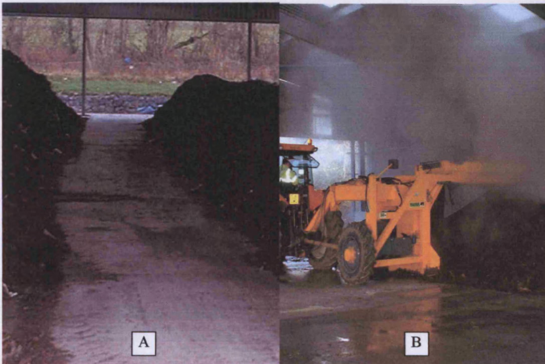
Figure 3.1. Windrows at the Composting Research Facility (A), and the windrow turner operating in the building (B).
