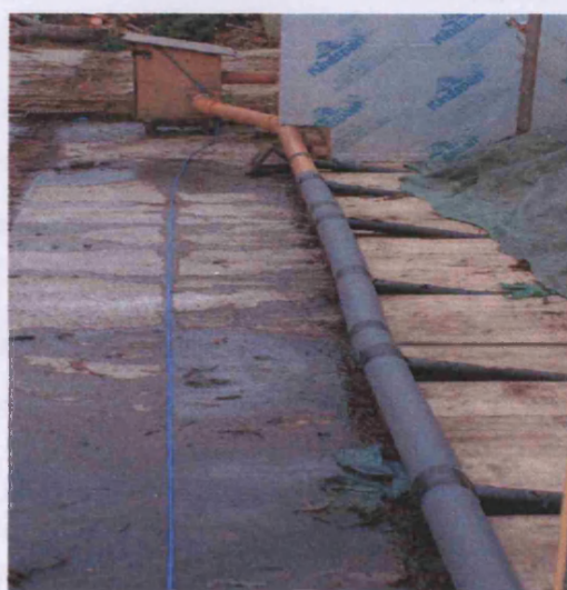
Figure 4.3 Aeration fan and manifold connected to perforated distribution pipes.
