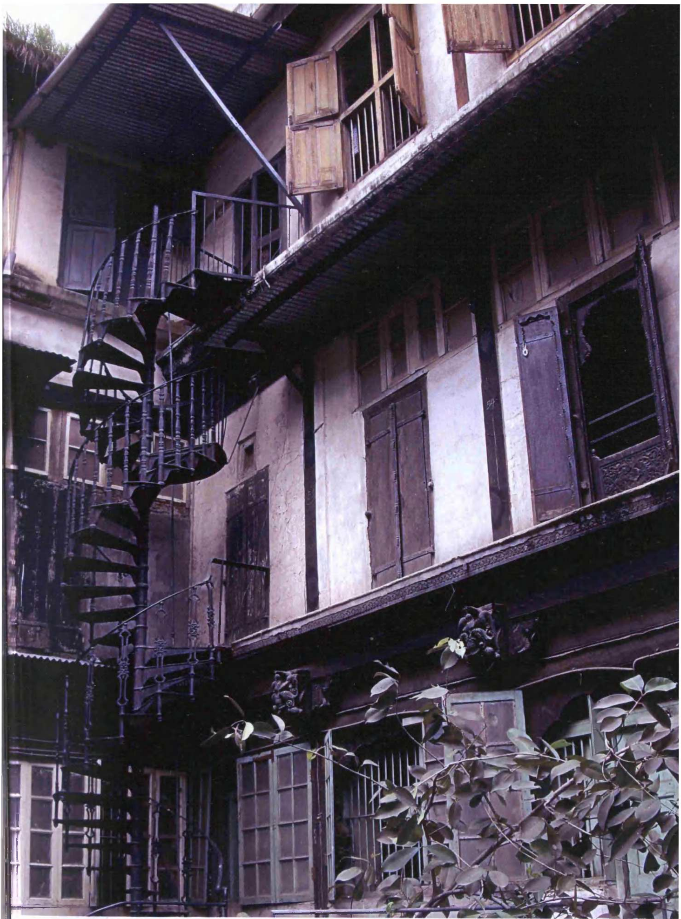
Fig. 8.121: Vishrambagh Wada, Pune, originally built: c.1803, Taluka: Pune, Zilla: Pune, Region: Desh, first internal courtyard
