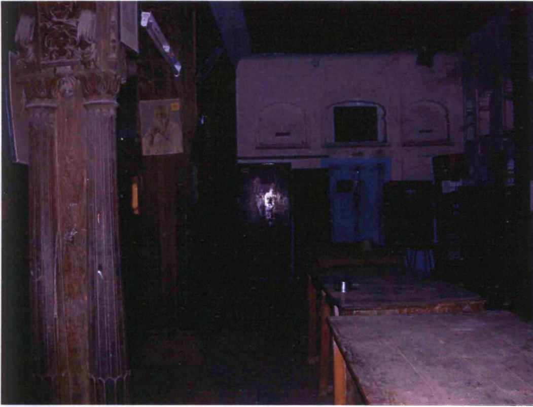
Fig. 8.42: Holkar Wada, Vafgaon, originally built: c.1725, Rajgurunagar, taluka: Khed, Zilla: Pune, Region: Desh, rangmahal first floor
