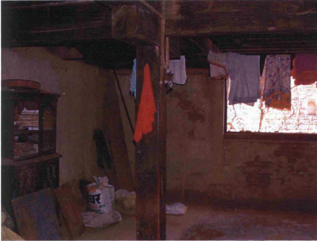
Fig. 8.68: Purandhare Wada, Modwa, originally built: c.1700, Taluka: Baramati, Zilla: Pune, Region : Desh, interior
