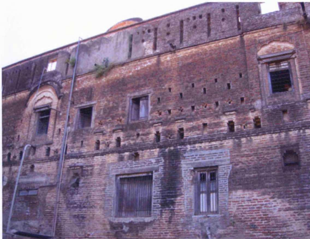
Fig. 8.21: Holkar Wada, originally built: c.1760, Chandwad, Taluka: Chandwad, Zilla: Nasik, Region: Desh, rear elevation showing composition of openings
