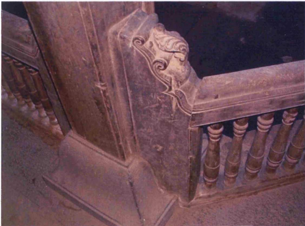
Fig. 8.133: Senapati Mohite Wada , originally built: c.1700, Rajewadi, Taluka: Khandala, Zilla: Satara, Region: Desh, wooden railing detail
