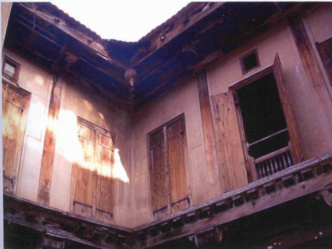
Fig 8.174: Menavli Wada, originally built: c.1768, Menavli, Taluka:Wai, Zilla: Satara, Region:Desh, view of the upper floor from the internal courtyard
