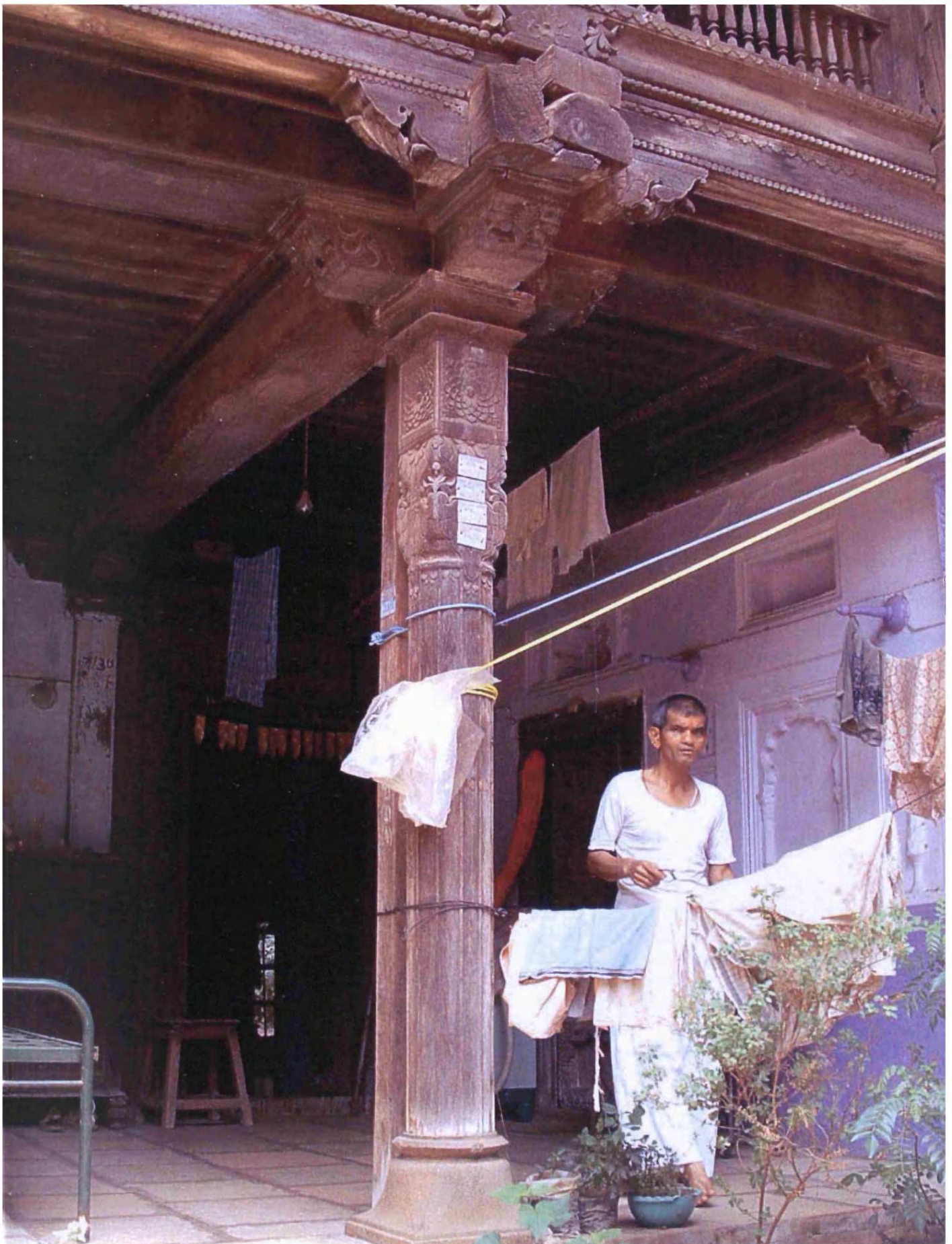
Fig. 8.143: Datar Wada, originally built: c.1725, Taluka: Pen, Zilla: Raigad, Region: Konkan, wooden column and beam supporting wooden ceiling
