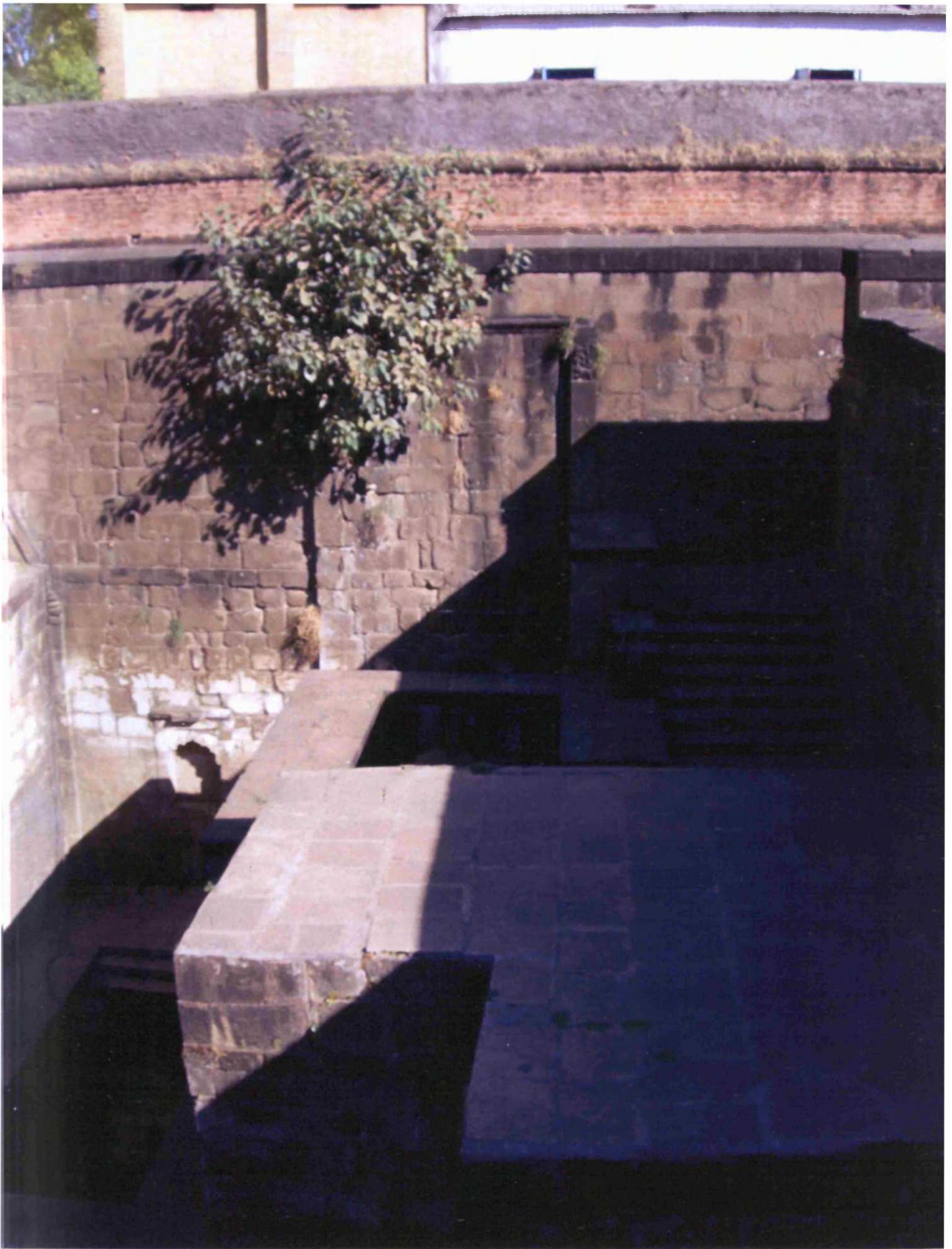
Fig. 8.24: Holkar Wada, originally built: c.1760, Chandwad, Taluka: Chandwad, Zilla: Nasik, Region: Desh, steps leading to water tank in the rear
