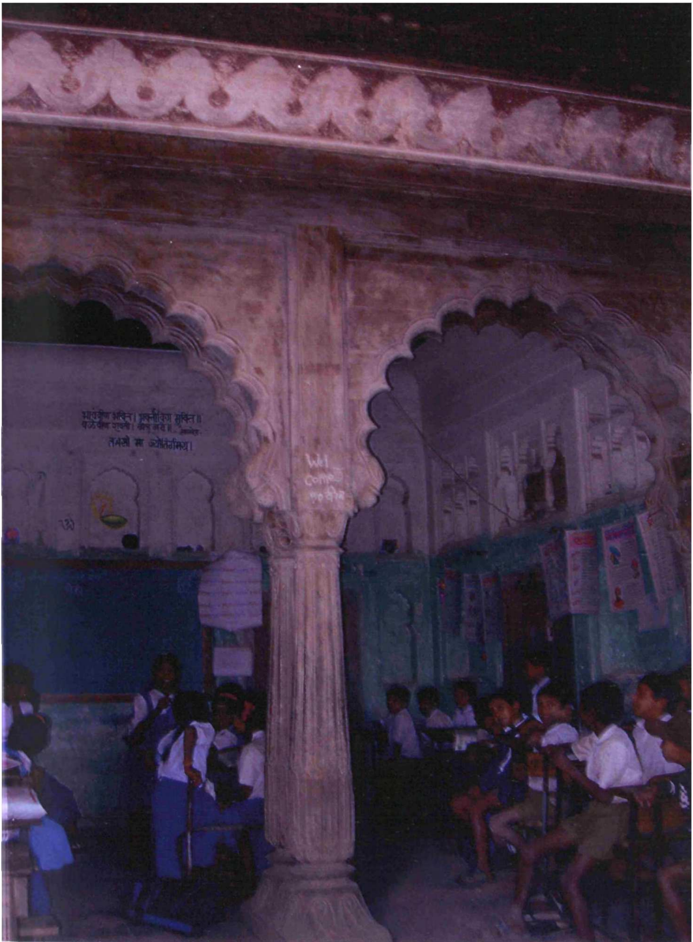
Fig. 8.45: Holkar Wada, Vafgaon, originally built: c.1725, Rajgurunagar, taluka: Khed, Zilla: Pune, Region: Desh, rangmahal
