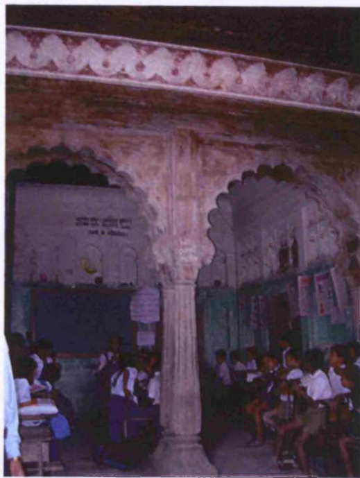
Fig. 2.5: Holkar Wada, originally built: c.1725, Vafgaon, Rajgurunagar, Taluka: Khed, Zilla: Pune, Region: Desh, rangmahal
