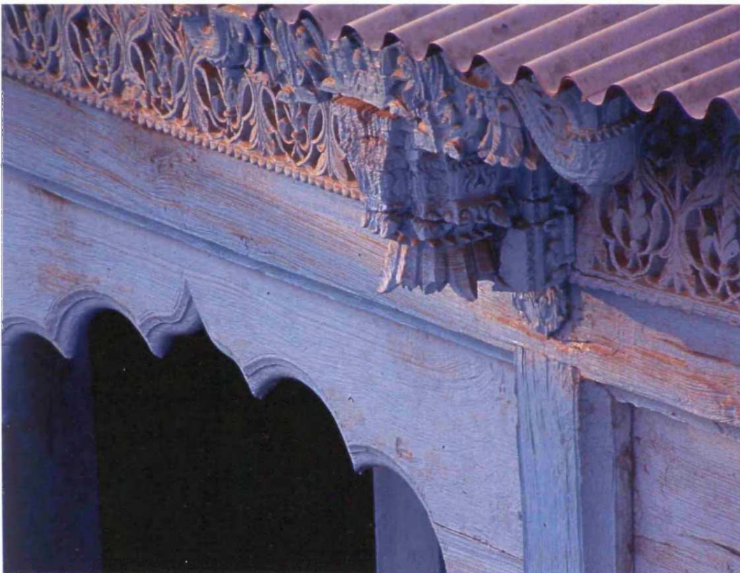
Fig 8.92: Mahadji Shinde Wada, originally built: c.1700, Taluka: Srigonda, Zilla: Ahmednagar, Region: Desh, detail of wooden arch and ornamental carving
