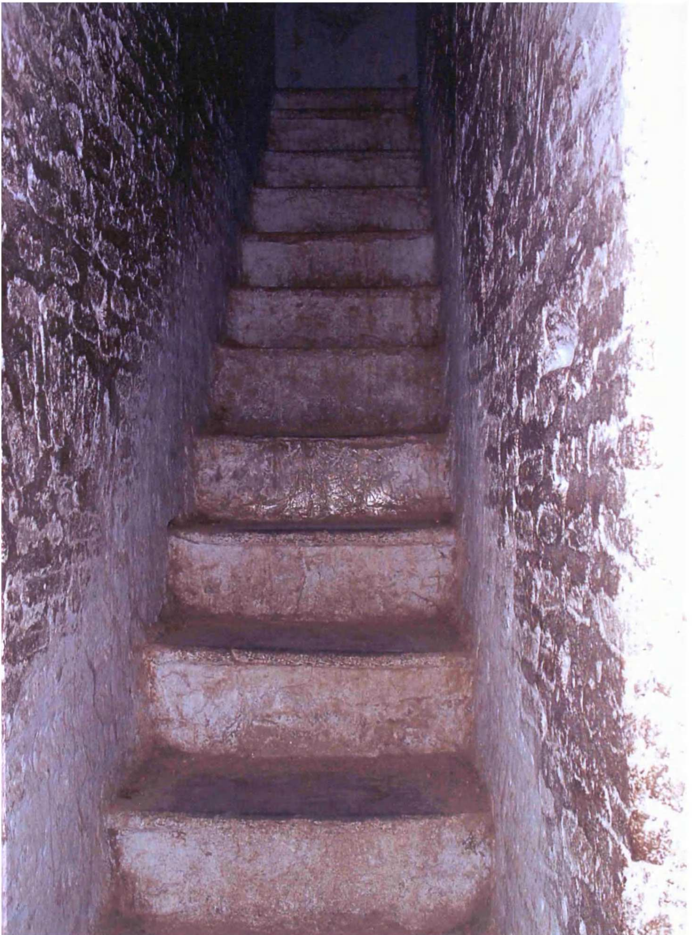
Fig 8.95: Mahadji Shinde Wada , originally built: c.1700, Taluka: Srigonda, Zilla: Ahmednagar, Region: Desh, staircase detail
