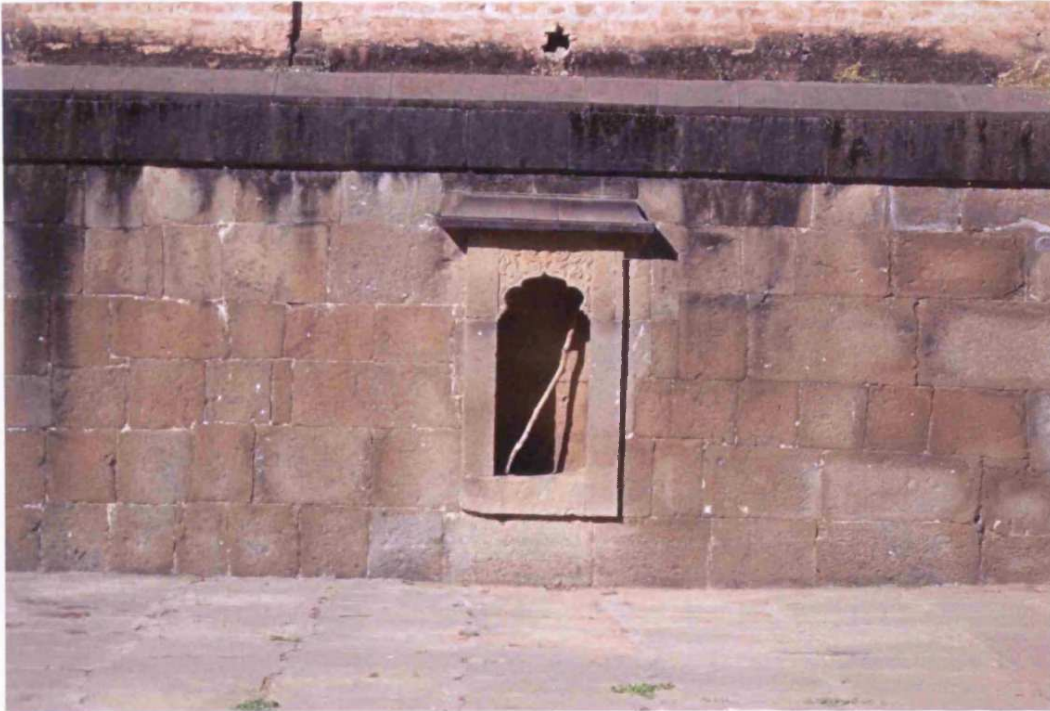
Fig. 8.26: Holkar Wada, originally built: c.1760, Chandwad, Taluka: Chandwad, Zilla: Nasik, Region: Desh, wall of stepwell
