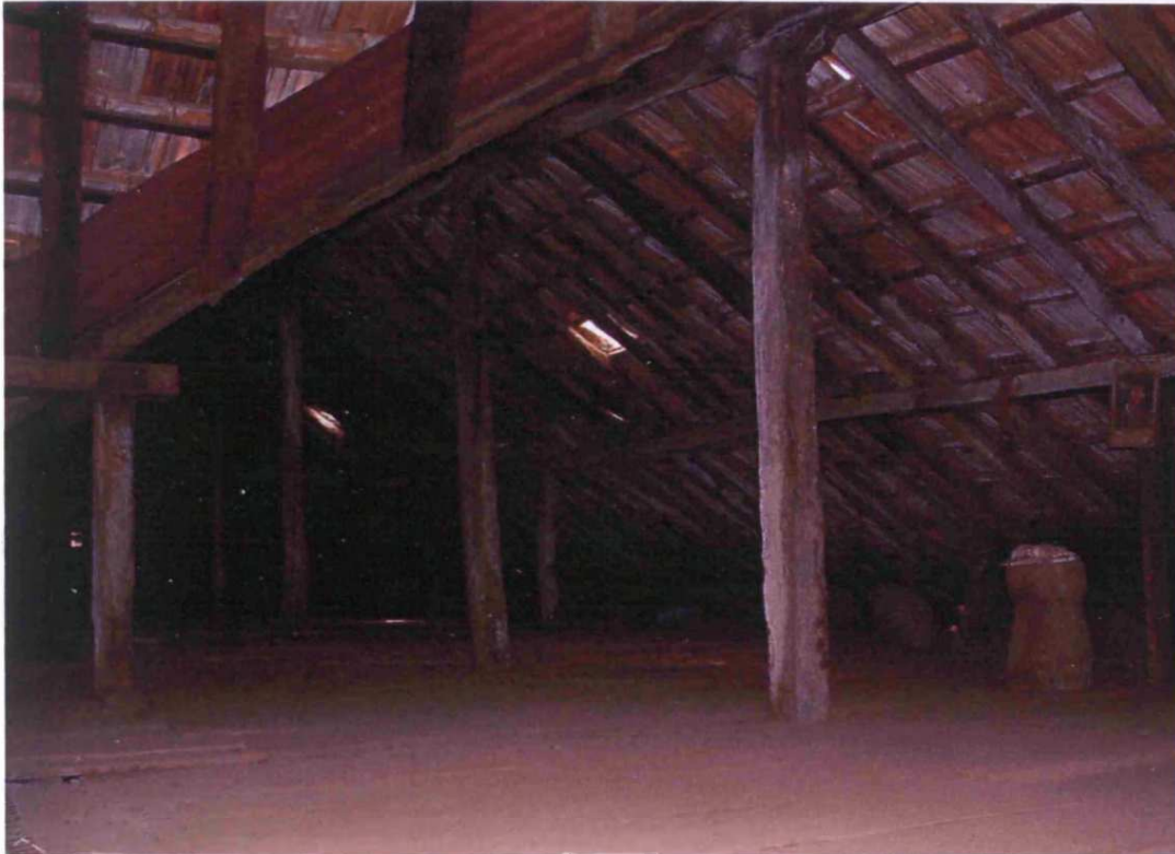
Fig. 8.141: Datar Wada, originally built: c.1725, Taluka: Pen, Zilla: Raigad, Region: Konkan, attic on second floor
