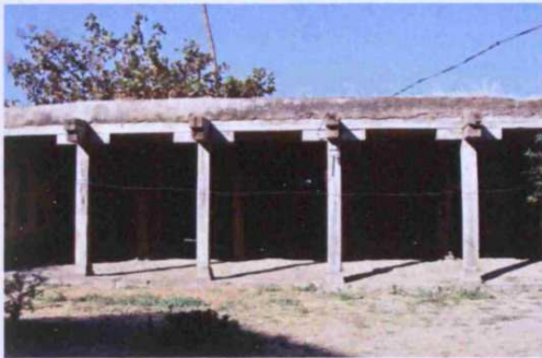
Fig. 4.12: Holkar Wada, originally built: c.1760, Chandwad, Taluka: Chandwad, zilla: Nasik, Region: Desh, Stables in the rear courtyard
