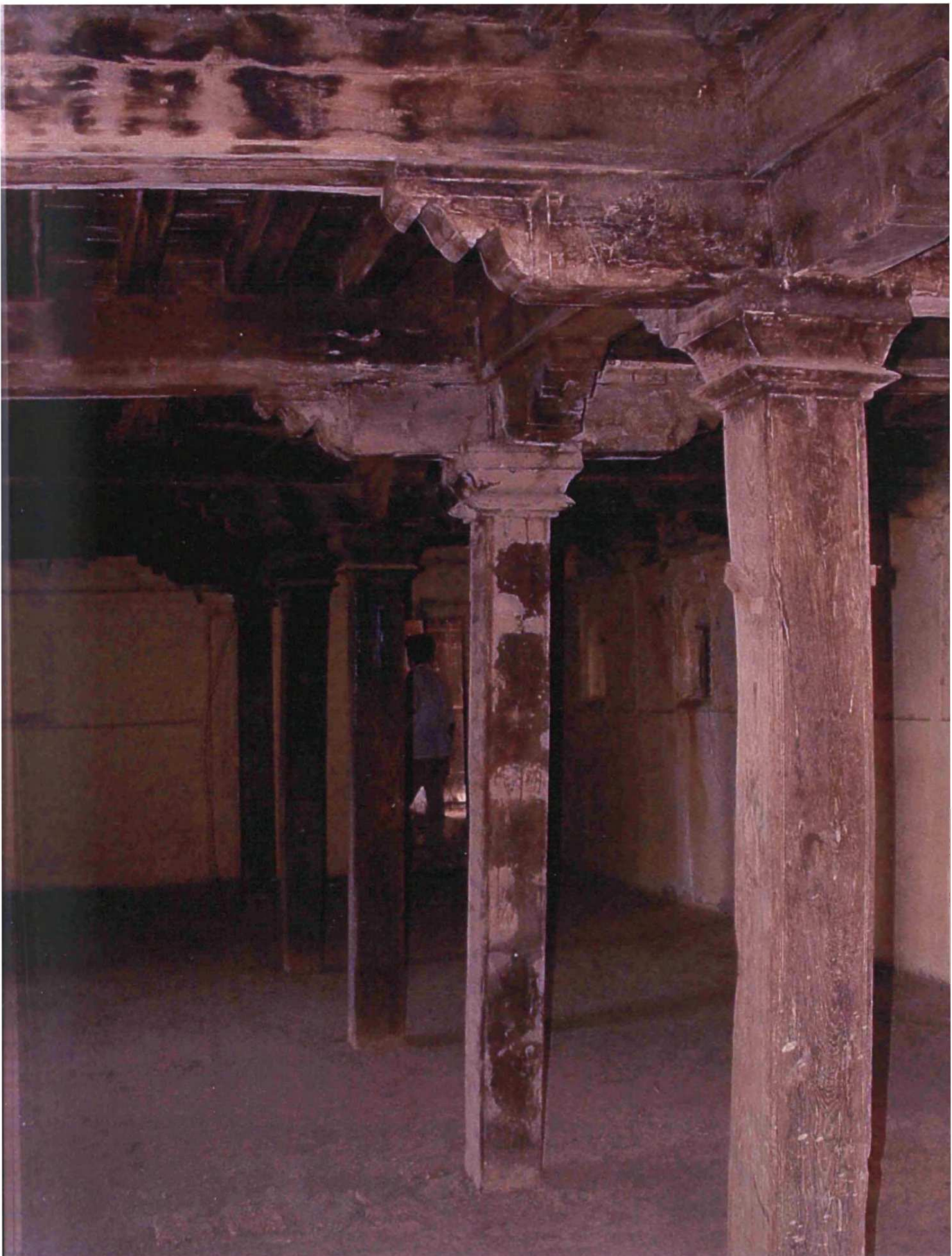
Fig. 8.54: Jadhav Rao Garhi, originally built: c.1600, Taluka: Purandhar, Zilla: Pune, Region: Desh, view of sofa with wooden columns, beams and ceiling
