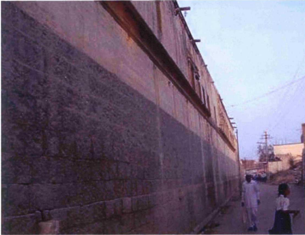
Fig 8.86: Mahadji Shinde Wada , originally built: c.1700, Taluka: Srigonda, Zilla: Ahmednagar, Region: Desh, exterior view from street
