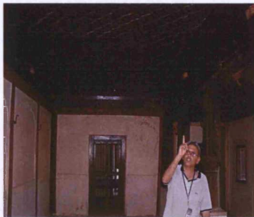
Fig. 4.1: Phadnis Wada , originally built: c.1738, Menavli, Taluka: Wai, Zilla: Satara, view of the diwankhana
