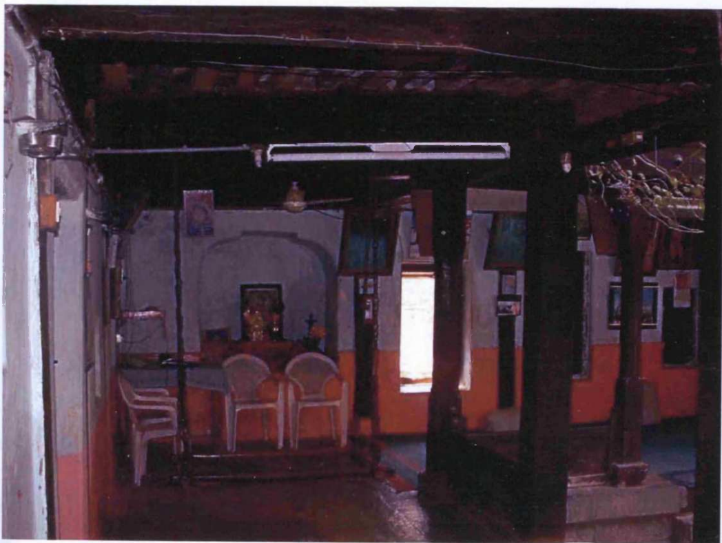
Fig. 8.154: Patil Wada, originally built: c.1700, Taluka: Paithan Zilla: Aurangabad, Region: Marathwada, sofa abutting internal court
