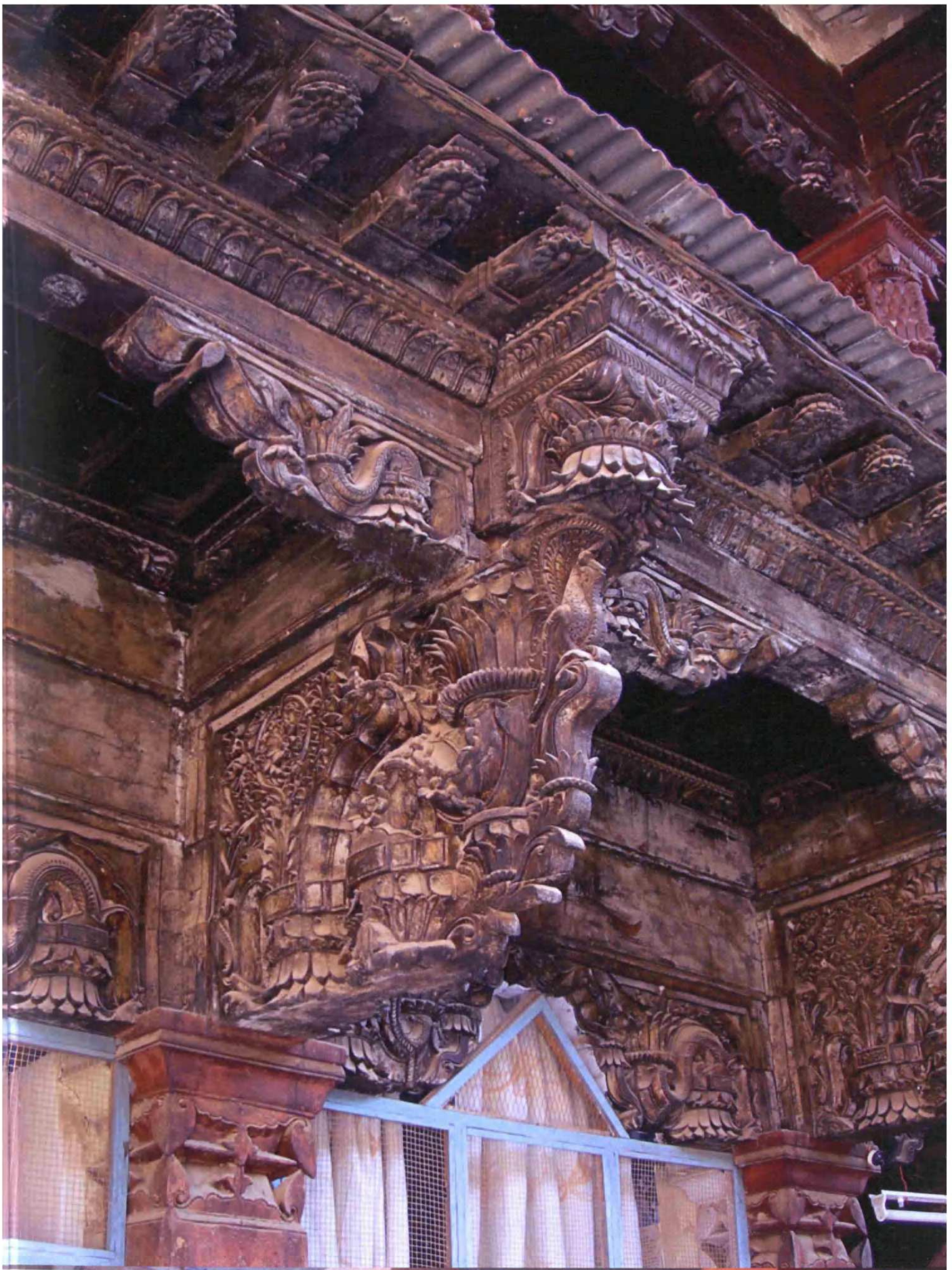
Fig. 8.18: Holkar Wada, originally built: c.1760, Chandwad, Taluka: Chandwad, Zilla: Nasik, Region: Desh, bracket and beam detail
