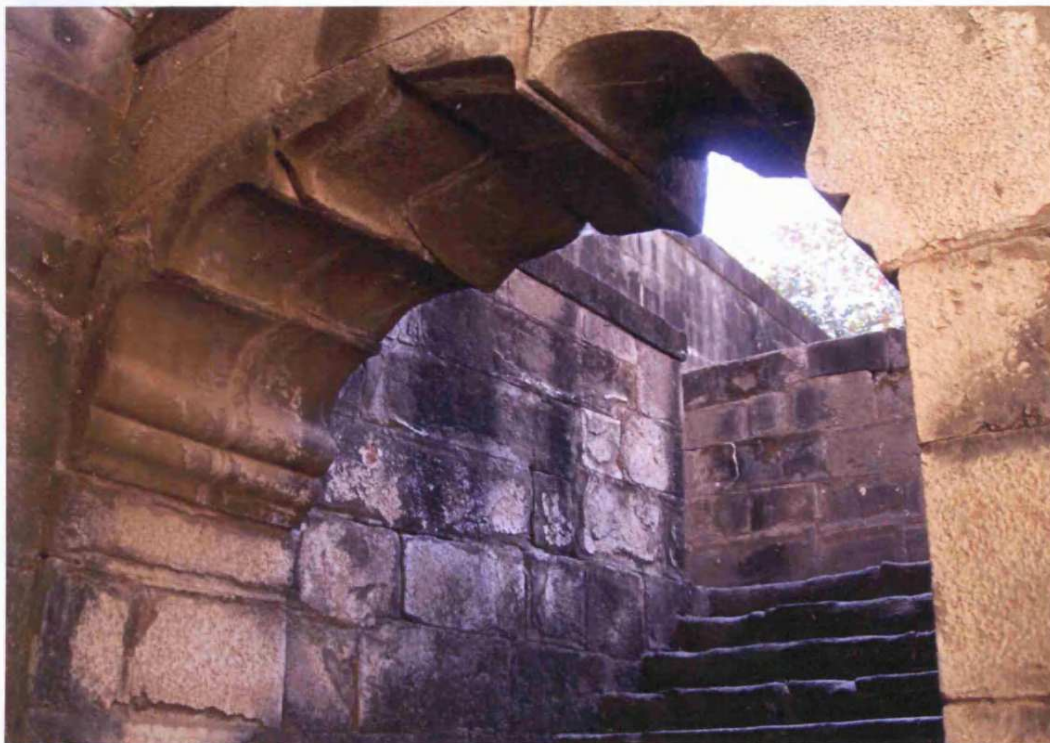
Fig. 8.27: Holkar Wada, originally built: c.1760, Chandwad, Taluka: Chandwad, Zilla: Nasik, Region: Desh, stepwell arch
