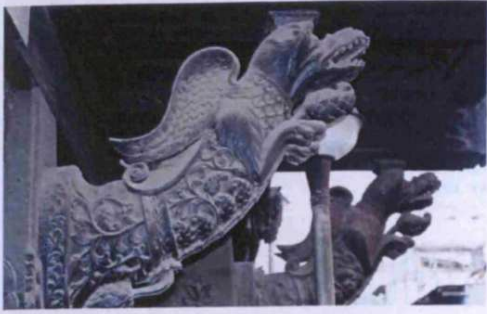
Fig. 2.4: Vishrambagh Wada, originally built: c.1803, Pune, Zilla: Pune, region: Desh, bracket detail
