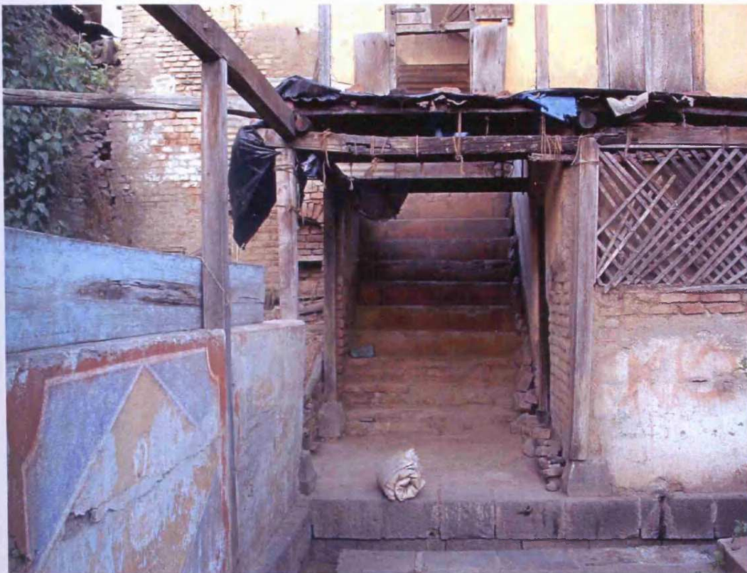
Fig. 8.197: Goshale Raste Wada, Wai, originally built: c.1770, Taluka:Wai, Zilla: Satara, Region: Desh, stairs leading on to the first floor used by cattle
