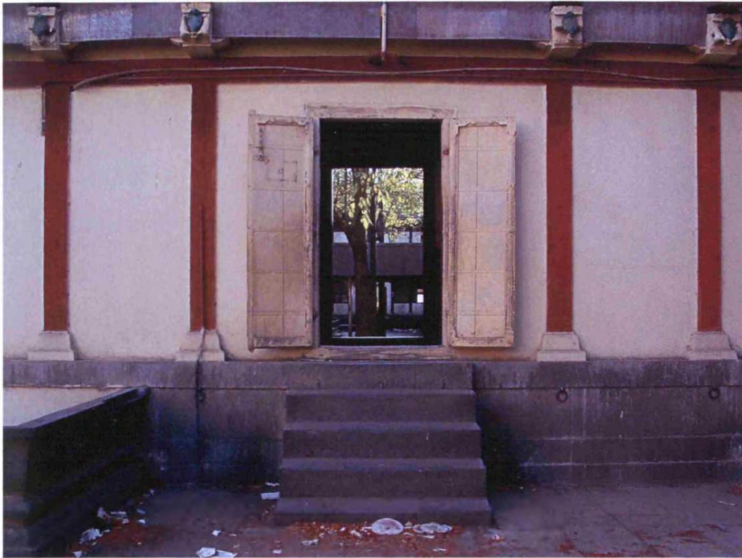
Fig. 8.113: Rajwada , originally built: c.1700, Taluka: Satara, Zilla: Satara, Region: Desh, built form between courtyards
