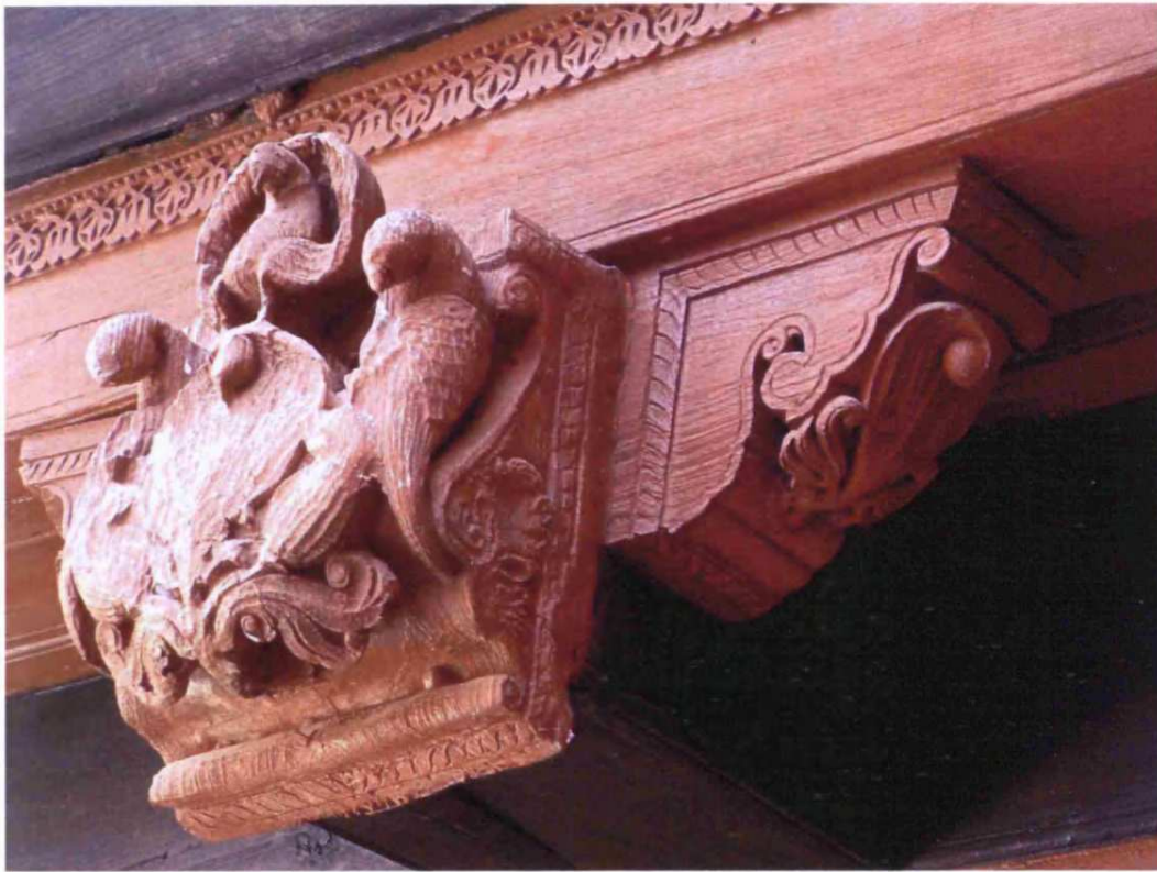
Fig. 8.80: Kadam Wada, originally built c.1700, Taluka: Mulgaon, Zilla: Satara, Region: Desh, detail of beam head
