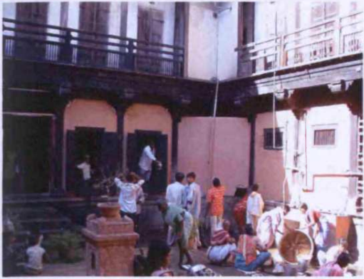
Fig. 3.30: Bhor Rajwada, originally built: c.1750, Bhor, Zilla: Pune, Tulsi Vrindavan, internal court
