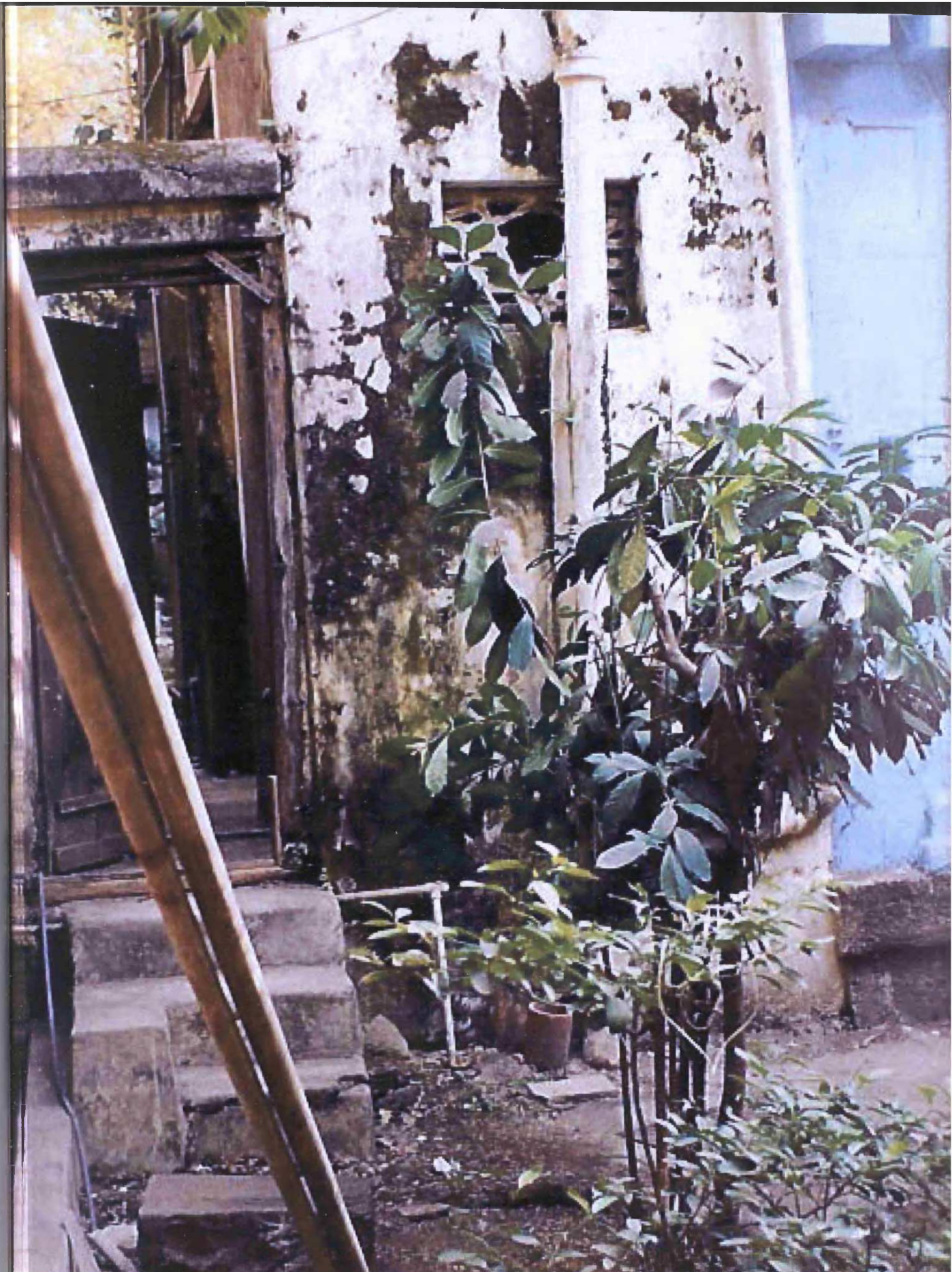
Fig. 8.151: Joshi Wada, Kalyan, originally built: c.1850, Old Kalyan, Taluka: Kalyan, Zilla:Thane, Region: Konkan, rear courtyard
