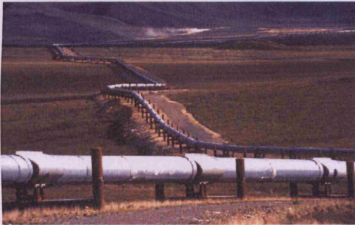
Figure 18: Above ground pipeline
