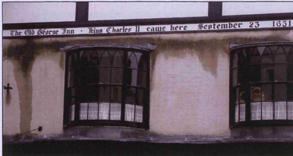
Figure 11 Wet facade in Bridport
