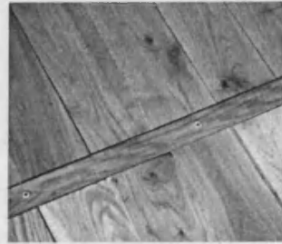
Timber floor showing the cover strip screwed to the subfloor with exposed fixings
