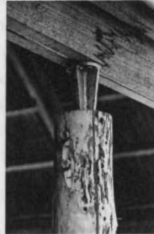
The timber sections of the covered entrance area are bolted or screwed to facilitate their dismantling
