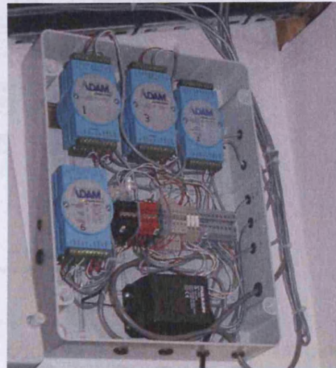
Figure A-2: Counter modules used in the monitoring [Advantech, 2006]
