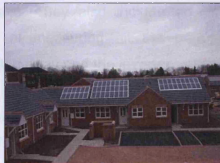
Figure 3-5: Building with building integrated photovoltaic at Nottingham
