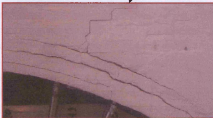
Plate 6-10: Arch condition after test (S3D-3R)
