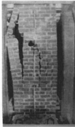
Figure 3-4 – Failure of a brick column
