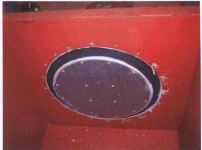
B 3.2 A view of the actuator plate taken from within the bath Note: The plate is not aligned with the inside of the bath because the water has been drained.
