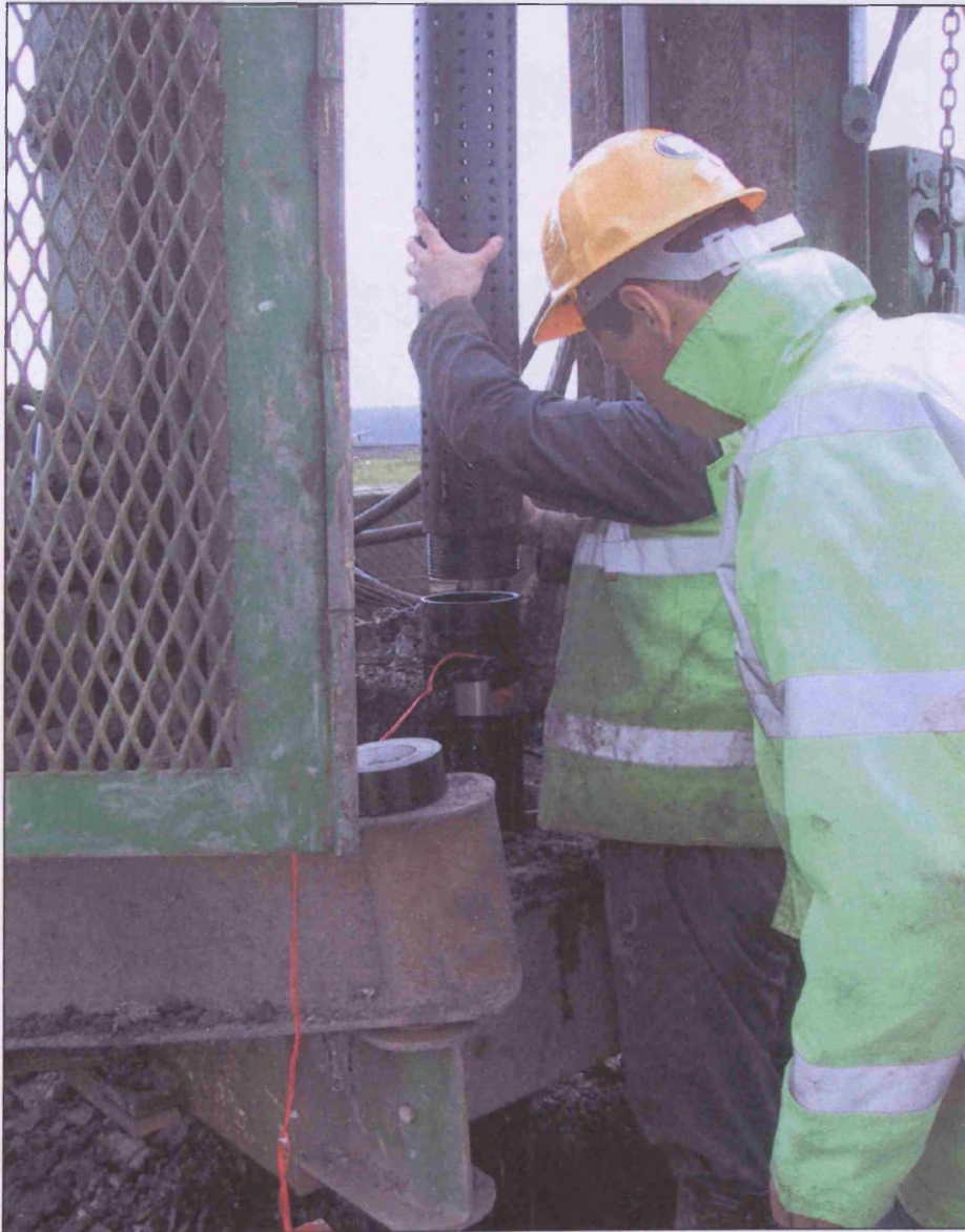
Figure 6.5: A photograph illustrating attachment of an electrode array onto the exterior casing surface during emplacement of a gas recovery well at Nantygwyddon (Jeremy Jones, Encia Consulting Ltd).
