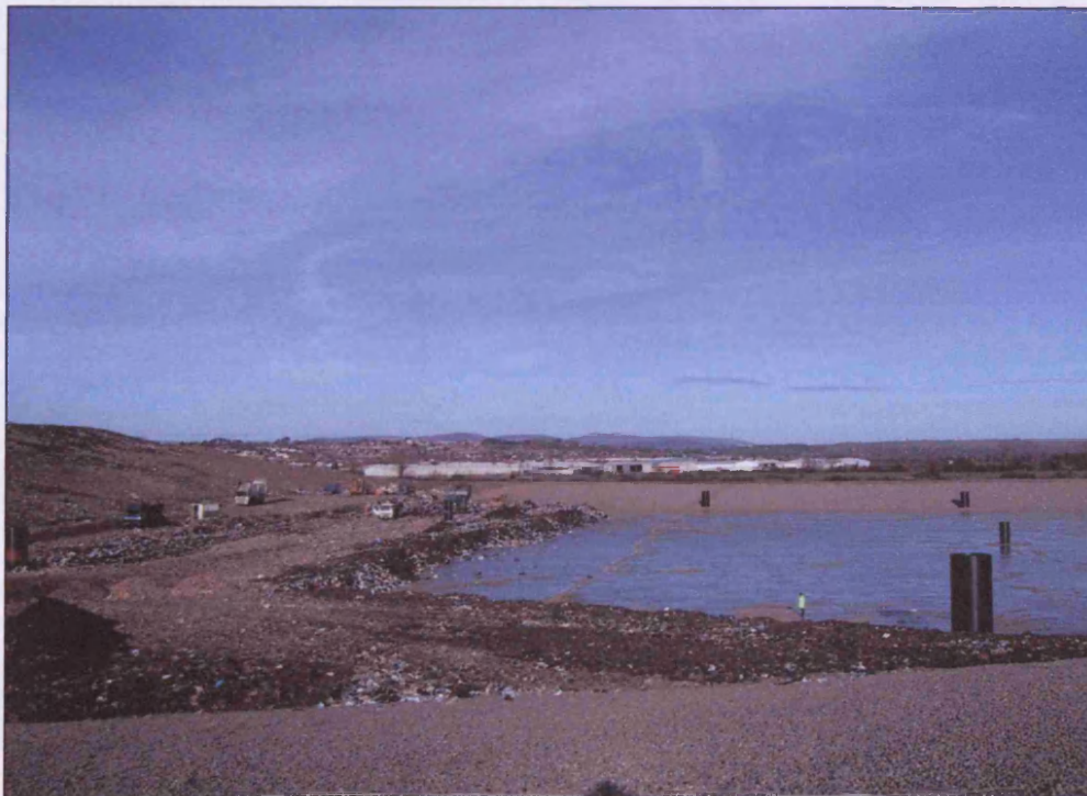
Figure 5.9: A photograph illustrating progressive burial of the electrode array by a series of refuse raises (author).
