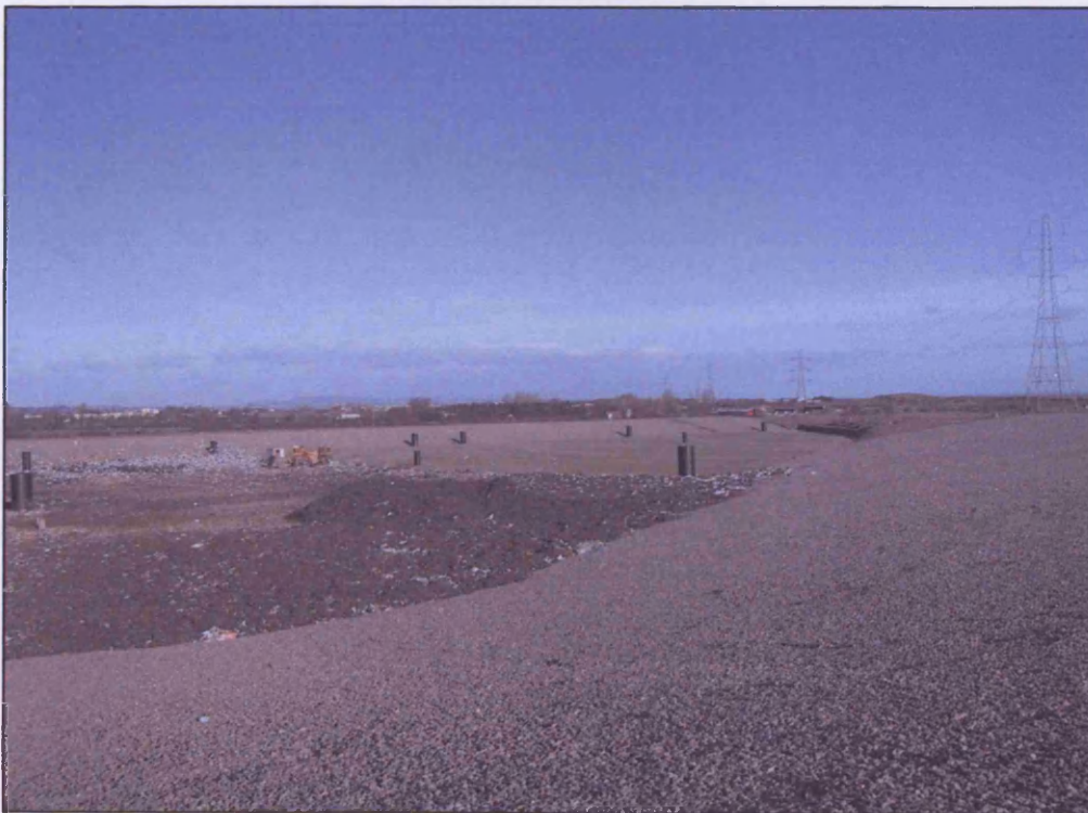
Figure 3.18: A photograph taken in March 2003 illustrating the start of refuse emplacement at Cell 2, Lamby Way (author).
