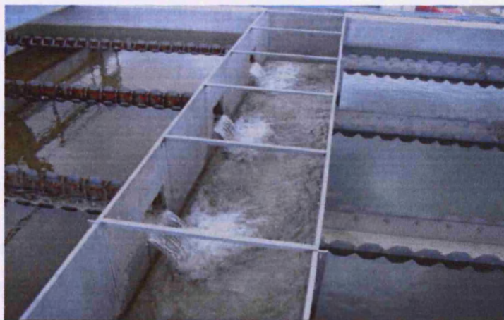
Figure 4.14: Wheal Jane MWTP clarifier overflow
